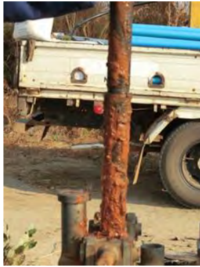
Corroded GI riser pipes (India Mark II hand pump)
