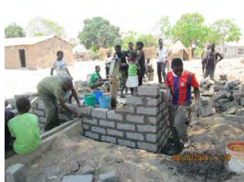
Community Installing Fence around Well fitted with Hand Pump (8th Oct, 2016 Milenge District)
