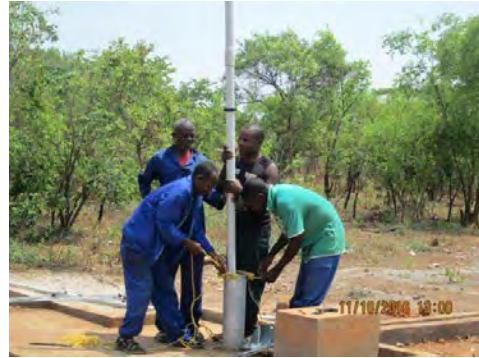
Installation of Hand Pump by APM on the Newly Constructed Well (11th Oct, 2016 Mwense)
