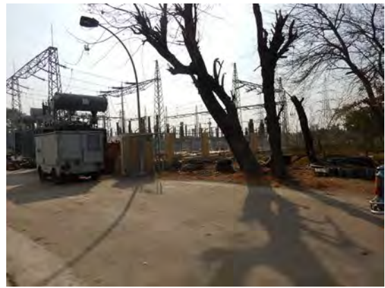
② Existing 132kV switch yard
