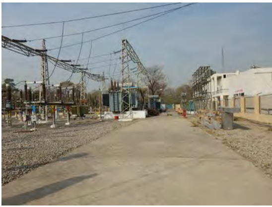
② Service corridor on side of 132kV switch yard
