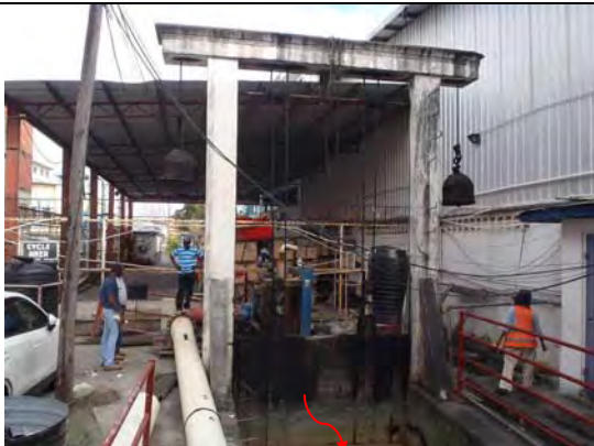
Church St. Sluice Gate and Mobile Pump
