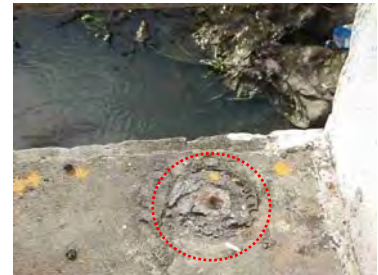
GT20 on Bridge across Church St. Channel. (GT20 is unavailable due to loss of steel rod)
