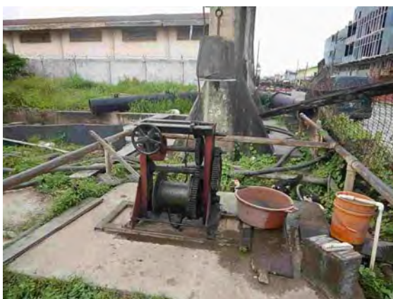
Wire Rope Winch Type (Princess St. Sluice)
