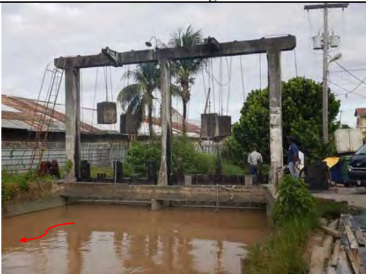
La Penitence South Sluice Gate
