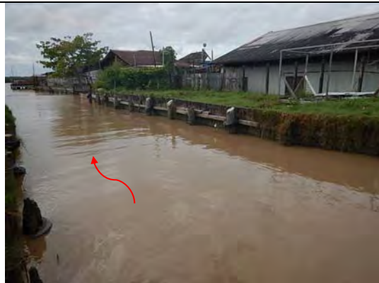
La Penitence South Drainage Channel
