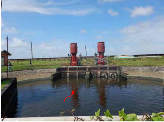
Liliendaal Pumping Station
