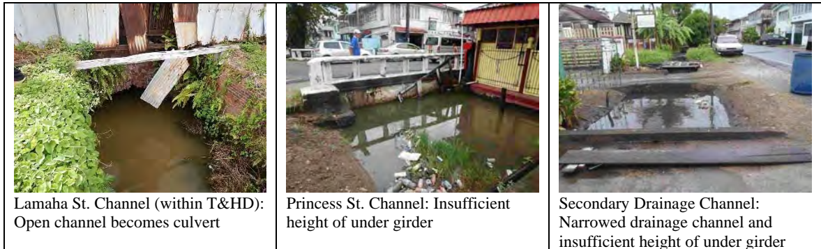
Photo R 2.1.1 Human-induced Interference and Narrowing of Drainage Channel
