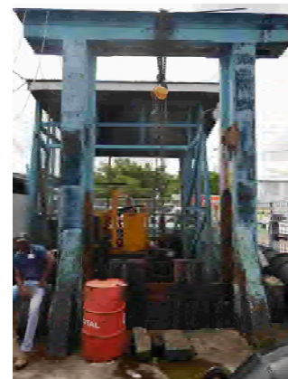
Chain Block Type (Commerce St. Sluice)
