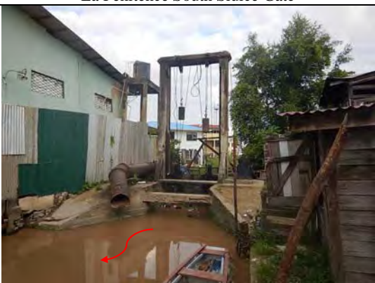
Ruimveldt North Sluice Gate
