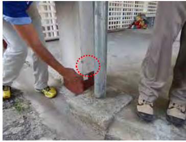
GT1 on Column of Court of Appeal Building
