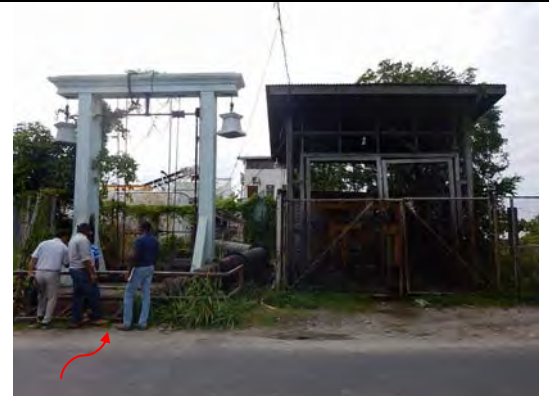
Lamaha St. Sluice Gate and Mobile Pump
