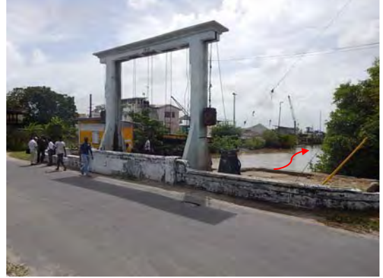
Cummings Sluice Gate
