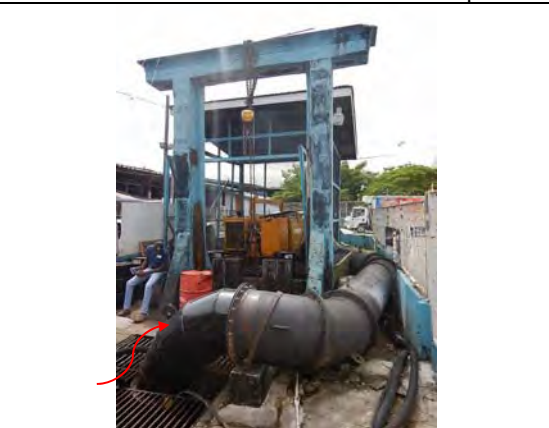
Commerce St Sluice Gate and Mobile Pump
