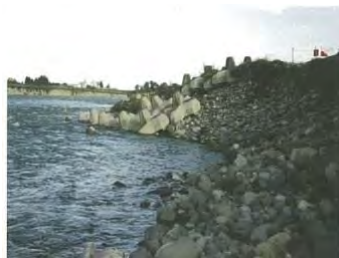
River bank erosion at the curved reach
