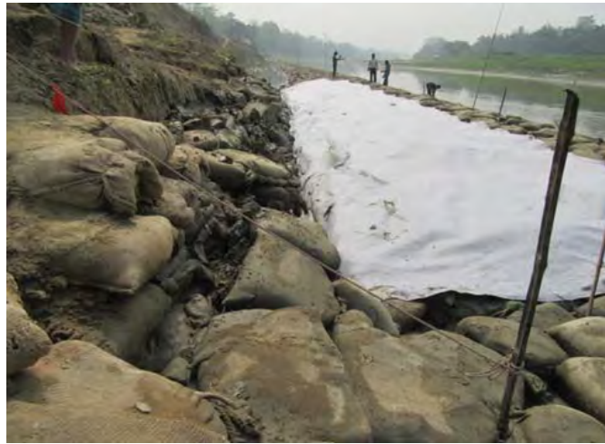
Ph11. Additional Geo-Textile sheets laid on S-C GB mound (inner half part of mound). @2016.02.16
