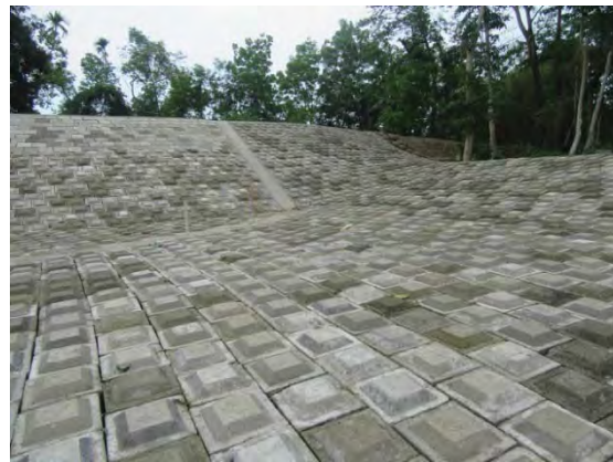
Placing of C.C. block with projection at Pilot Project site in Moulbvibazar
