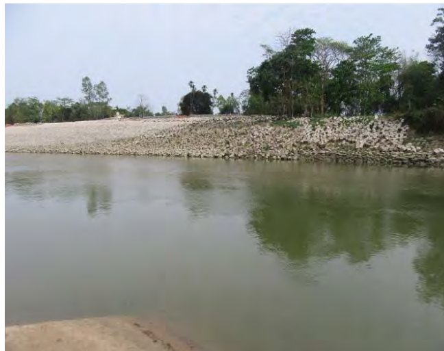
Ph35. View of up-stream, connection of PRW up-stream with the up-stream temporary protection. Taken from opposite bank @2017.03.09
