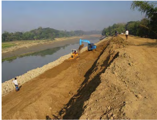
Ph24 *Down-stream lower slopes are preparing and compacting by bulldozer and excavator. @2017.01.22
