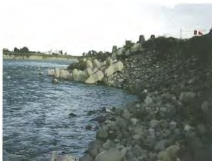
River bank erosion at the curved reach
