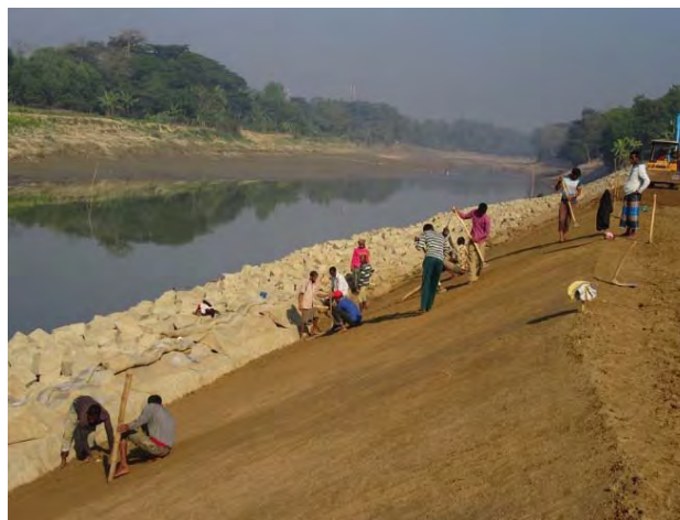
Ph25 At up-stream/ original soil area, lower slope of embankment are preparing by cutting and filling with compaction by 7 kg hammer. @2017.01.22
