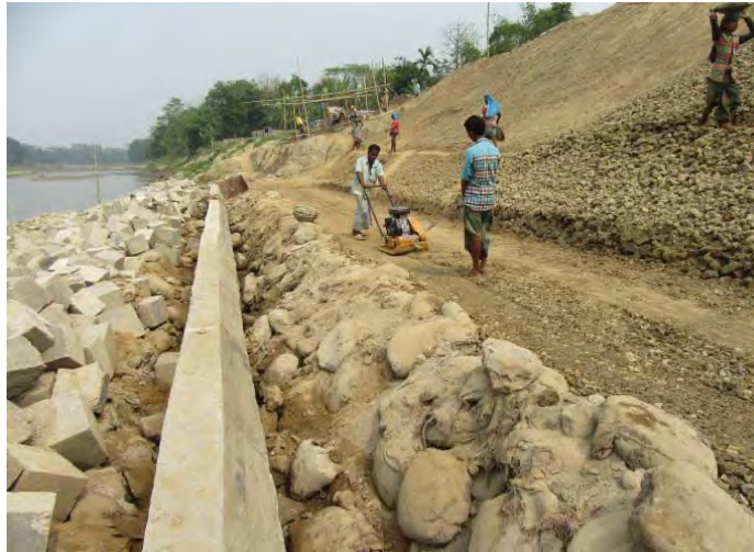
Ph13. On embankment river side slope ch. 10 – 30m, RL 6.00m(PWD) base preparation is running by plate compactor for layer by layer filling and compaction.@2016.03.11
