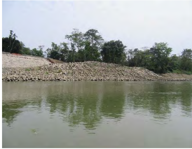
Ph34. View of up-stream, connection of PRW up-stream with the up-stream temporary protection. Taken from opposite bank @2017.03.09
