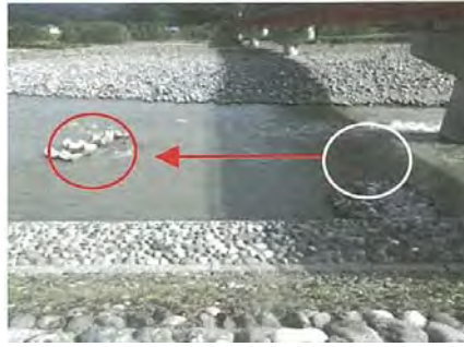
Figure 5.9 Outflow of Concrete Block of Groyne/Spur
