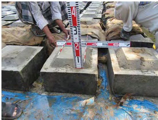
Manufacture of C.C. block with projection at Pilot Project site in Moulbvibazar
