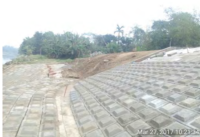
Ph33 Placing projection CC-blocks for Slope Protection and transition are in down stream. @2017.03.27
