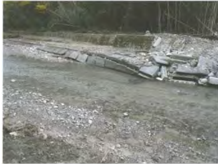
Deformation of foundation of bank protection by local scouring
