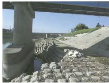
River bank erosion near a bridge pier
