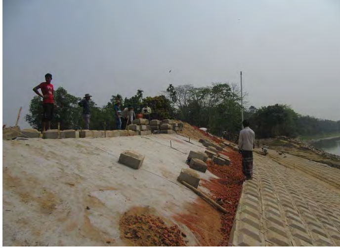
Ph30 Elevation level of 11.65m (DHWL) on the top of projected cc blocks on 2nd slope checked – found ok. @2017.03.1
