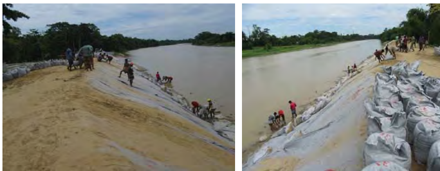
Ph22 & 23. Carrying of geo-bags and placing of geo-bags on toe of TPW (intermediate berm at around 9.00 m(PWD)) @2016.06.10 WL = 9.05 m
