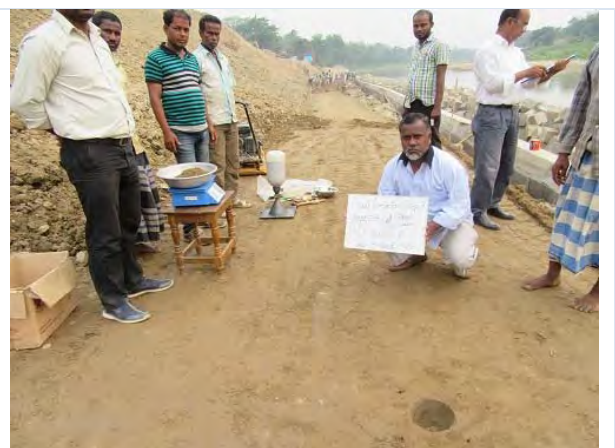
PhH. Field Density (FD) Test by sand-replacement method for test a) area ; 2 passes compaction by bulldozer plus one pass compaction by Plate Compactor
