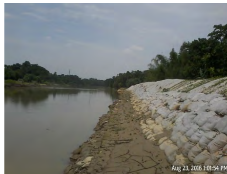
Condition of the slope during monsoon season @2016.08.23
