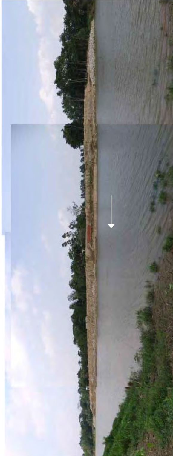
Photograph: Overall View of Pilot Repair Works (from the opposite bank on 21/Apr/2016)
