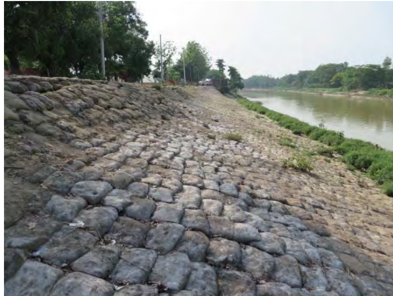
Photo 4.1.1 With sand-cement gunny bags Slope Protection on the left bank of Manu River, Moulvibazar
