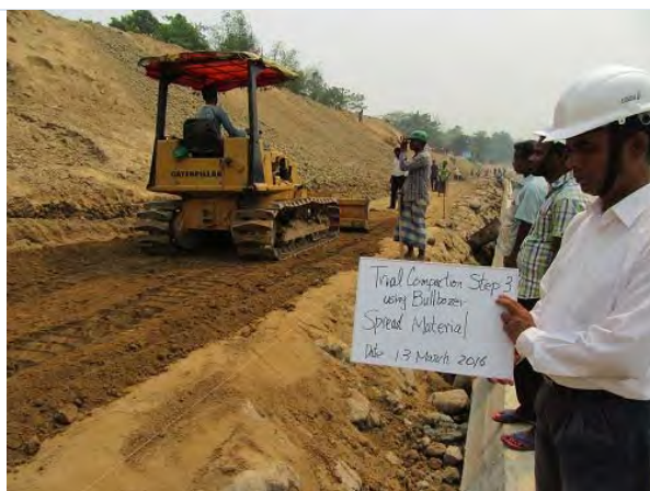
PhG. Spreading material by bulldozer by layer by layer, until loose thickness 25 cm
