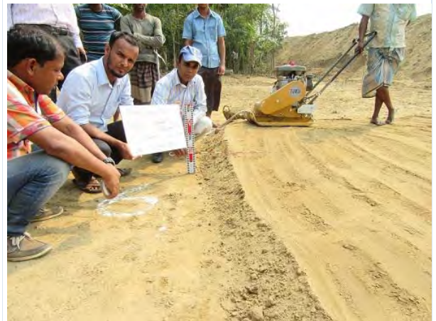
PhB. Step1(using "Plate Compactor"); compaction and check thickness after 2 passes of compaction
