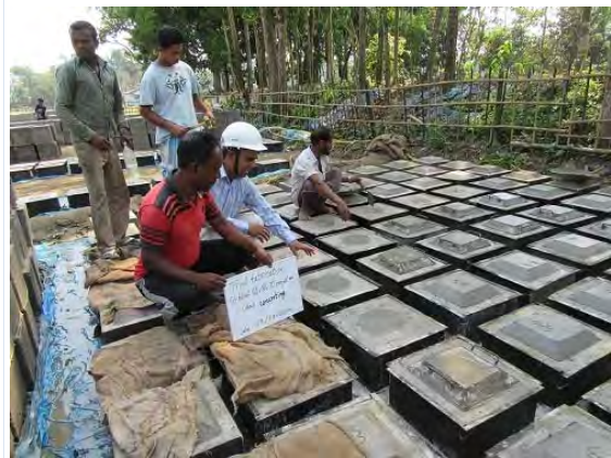
PhB. Scratching the surface and cement mortar plastering before casting projection part
