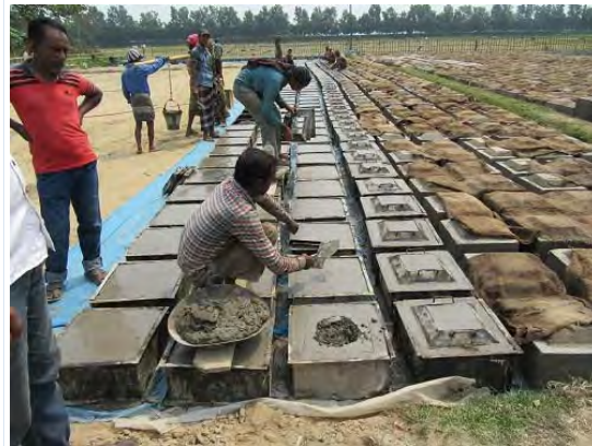
PhF. Doing room for improvement increasing adhesion between lower/upper part, make a hole at the lower part
