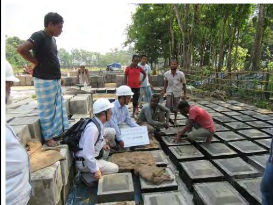
PhC. Checking the procedure of casting concrete and workmanship of manufacturing for projection part
