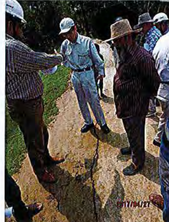
Ph4. Checking cracks on to the crest of the bank at about C/S # No.17
