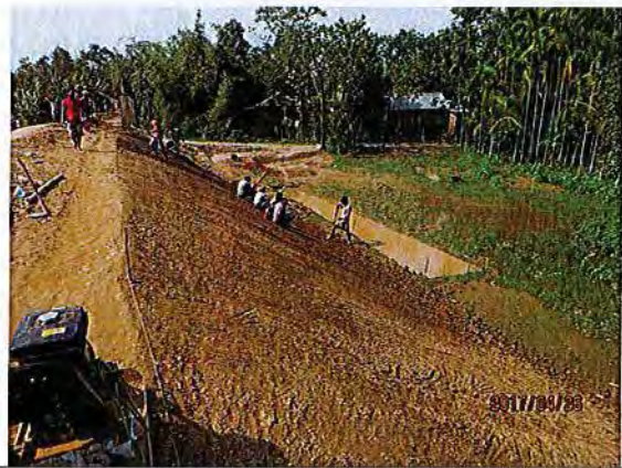
Ph2. Proposed Drainage at Toe of proposed country side slope. Existing swamp small ponds.
