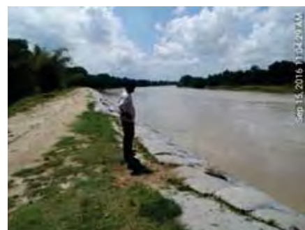
Photo 3.2. River water level of 11.00m (PWD) marked highest on this season on site. From down-stream to up-stream 15 Sept 2016.
