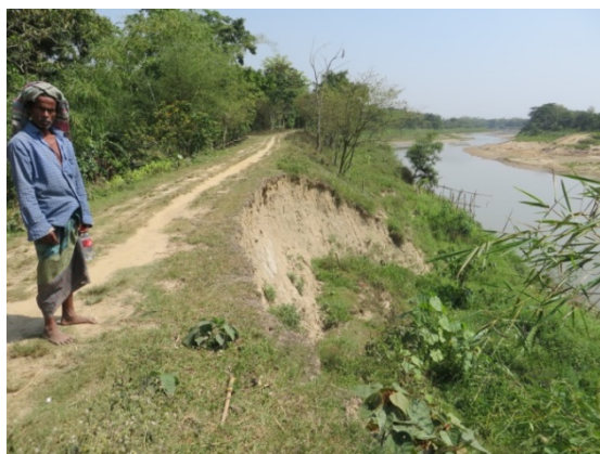
Photograph-3: Damaged Embankment (Moulvibazar: D-category)
