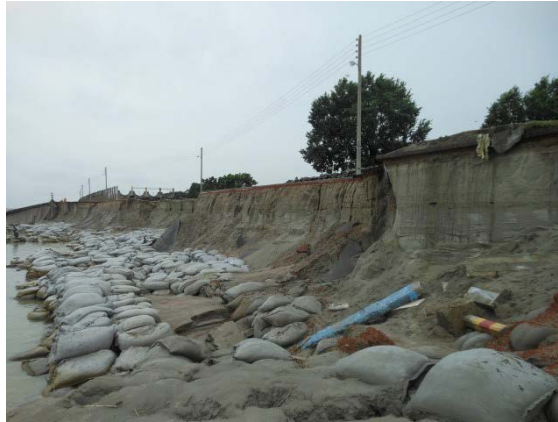
Photograph-1: Embankment failure (Sirajganj)
