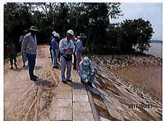
Ph5. Checking construction joint between placing cc-block on cracks and Gap concrete at about C/S # No.16
