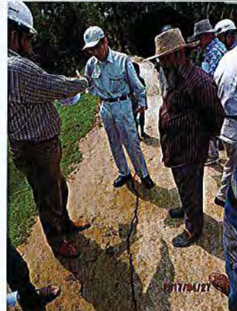
Ph4. Checking cracks on to the crest of the bank at about C/S # No.17
