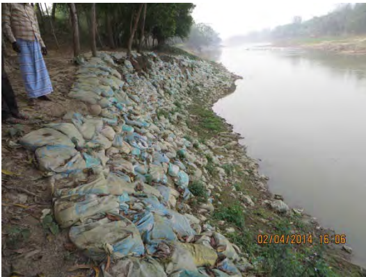
c. River bank eroded site
