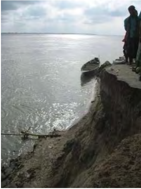
a. River embankment failure site
