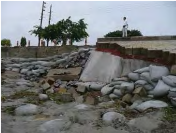
a. River embankment failure site
