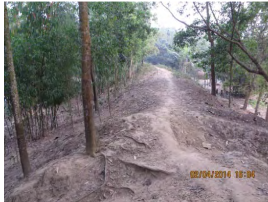
b. Damaged embankment due to the human traffic
