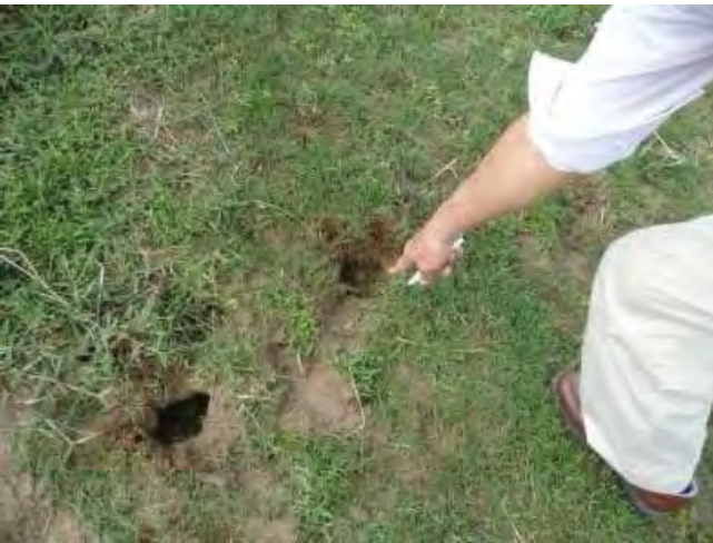
b. rat holes on the river embankment
