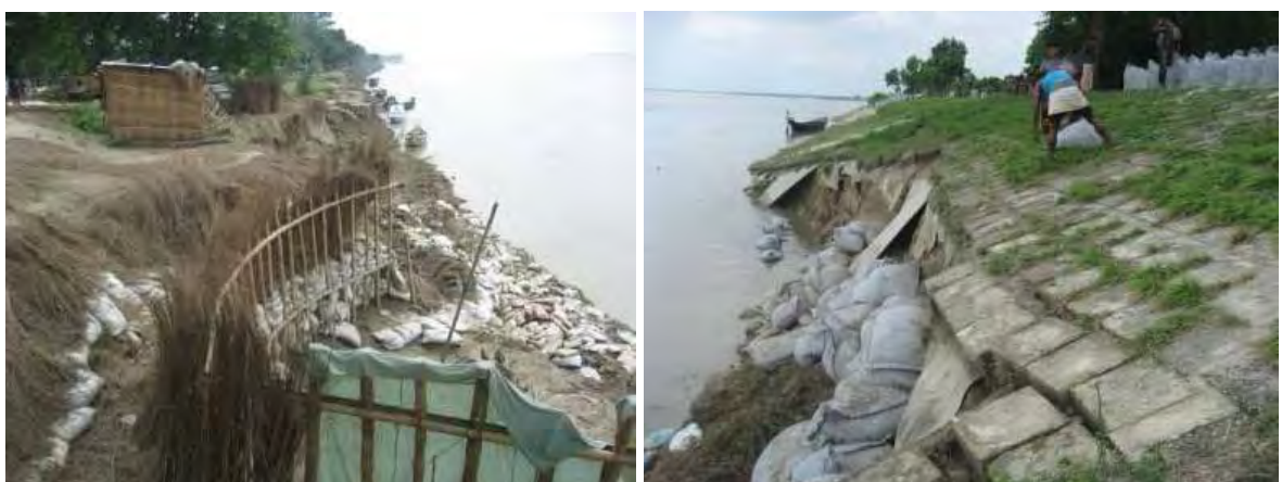
c. River Bank Erosion Site
