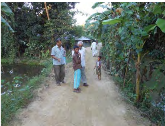
c. Sunken left embankment (the foundation layer may have a problem.)
