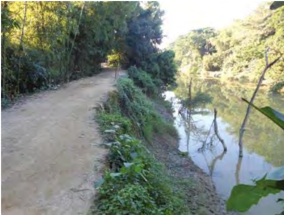
a. Eroded right embankment with the length of 300m. About 1/3 of the crown is lost.
