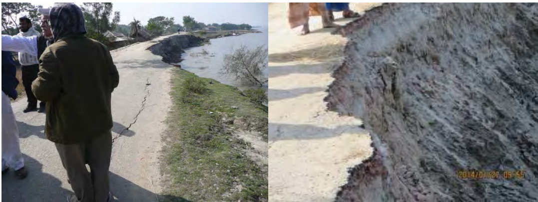
a. Embankment eroded site
