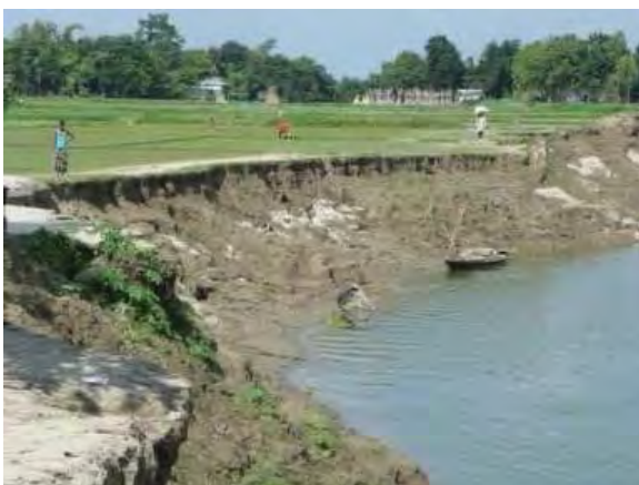
c. Embankment erosion on the city side in the downstream reaches of TPW.
