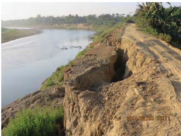
c. Damaged embankment due to the embankment toe erosion. Cracks are seen on the slope of the embankment and it is almost going to fall.
