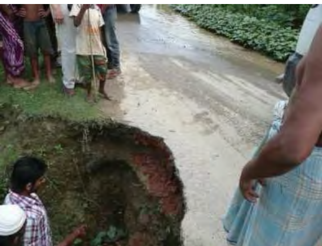
c. failure of river embankment
