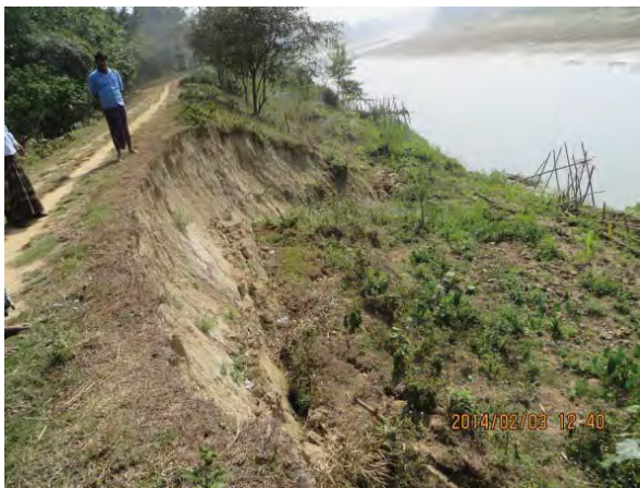
b. Due to the erosion at the embankment toe, the slope slide took place with the scale of 300m long. The embankment crown itself is already very narrow. There exists an elementary school nearby.
