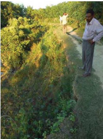
b. Eroded left embankment (about 1/2 of the crown is lost.)
