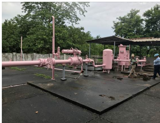
Photo-4 Gas Yard
