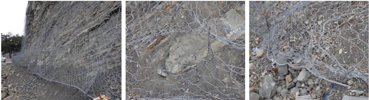
Fig. 2-2 Damage status of competitor’s products
