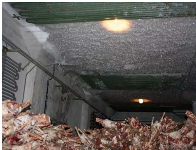
Figure 3.2.5 Frosted Refrigerator (indicative of low storage efficiency)
