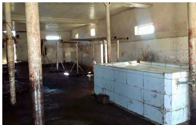
Figure 3.2.3 Small Slaughterhouse (note dirt and blood stains on walls and pillars)
