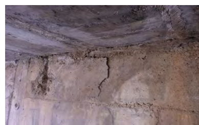
Spalling and re-bars exposures
