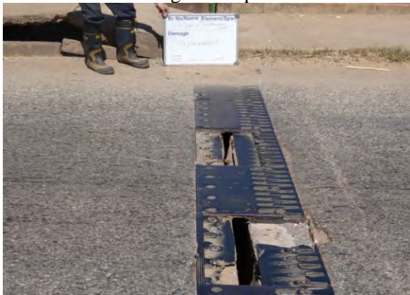
Damage on finger plate due to heavy traffic
