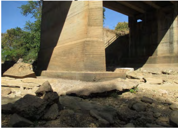
Scouring due to outflow of water or sand
