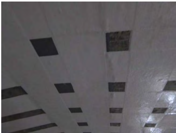
Carbon Fiber Sheet on Lower Surface of Slab (Metropolitan Expressway No.3 Route)
