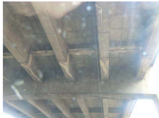
Damages of Bridge in Johannesburg City (Cracks, Water leakage, etc.)
