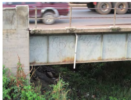
Another proposal; drain extension up to bottom flange with fabricated VP pipe and metal fitting
