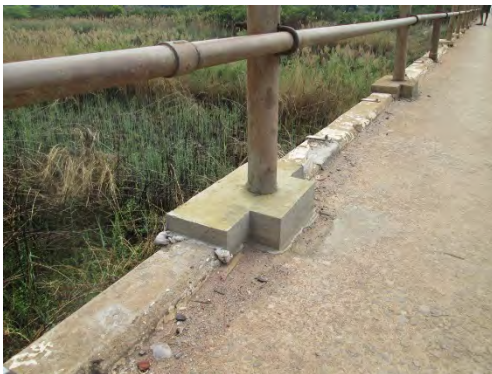
Repaired concrete member at a guardrail post base in the dry-run held on August
