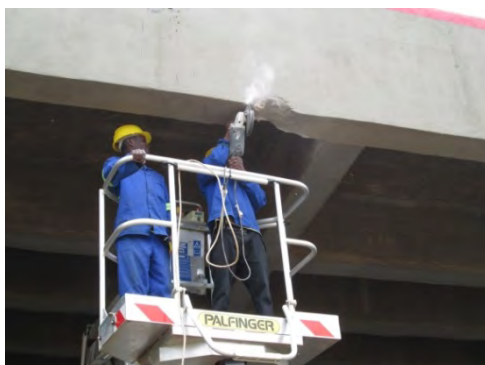
Patch repair to collision damage in concrete girders; close attention should be paid to the traffic under.
