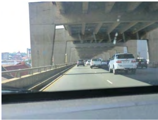
Damages of Bridge in Johannesburg City (Cracks, Water leakage, etc.)
