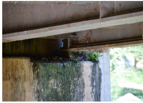
Water leakage from expansion joint
