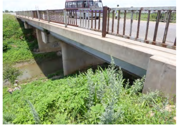
Paint peel-off and corrosion
