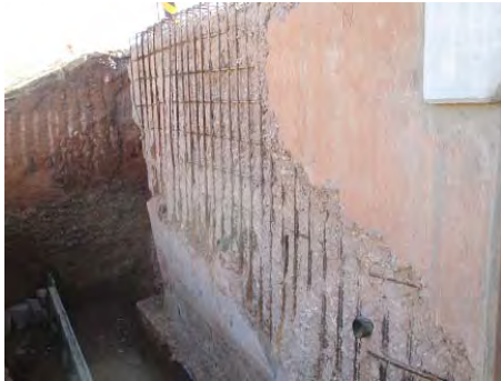
Damages on Wing of Bridge Abutment (Delamination of Concrete, Exposed Rebars)
