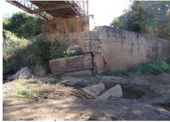
Damage on slope protection due to flood
