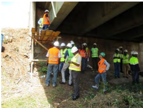
Site training: technical instruction for partial painting on the scaffolding built in front of abutment
