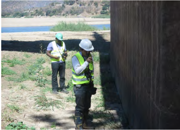
Vertical crack on the wall type pier
