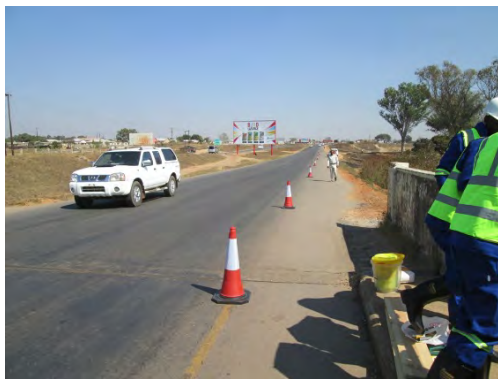
Dry-run at steel bridge on T3 Road over Kafue River. Traffic regulation completed.
