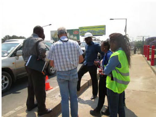
Technical instruction on site of concrete repairs; explaining the details of work procedures
