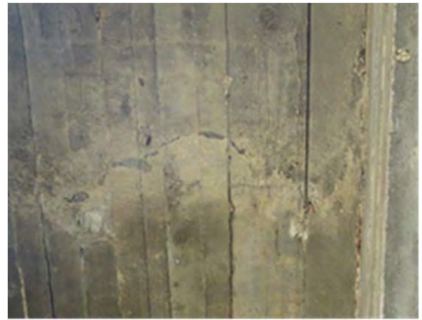
Deteriorated concrete surface
