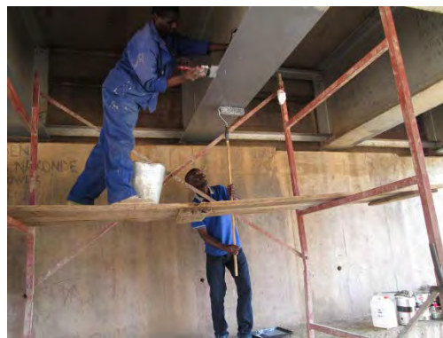
Applying epoxy primer coat using paint roller and brush with the installation of scaffolding
