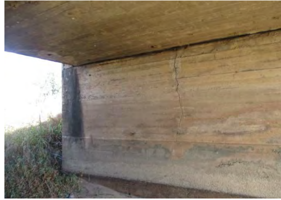
Vertical crack on front abutment
