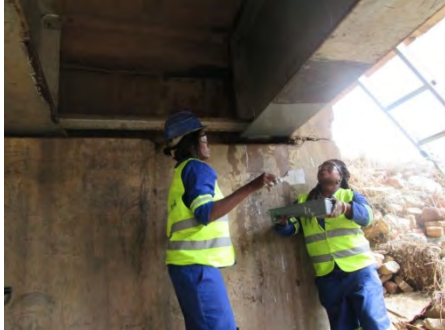
Preparation for Site training: primer application on lower flange of girder for touch-up paint
