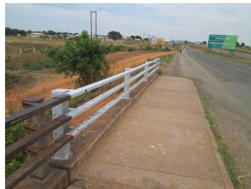
Repainted guardrail in the dry-run; unfortunately, many graffiti were already on it
