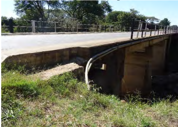
Damage due to car accident
