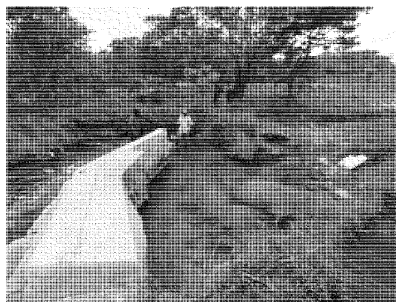
Simple weir (at front side) was constructed to reserve water (Chibolya Site, Kawambwa)
