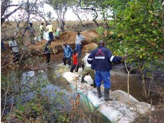
Construction of coffer dam: Constructing coffer dam with sand bags. MBL 2-7 Kawama. September 1, 2014
