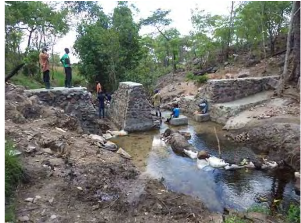
Upstream view of weir: Main part of stone masonry weir was completed. LWG 5-2 Mufili Chibwale. November 12, 2014.
