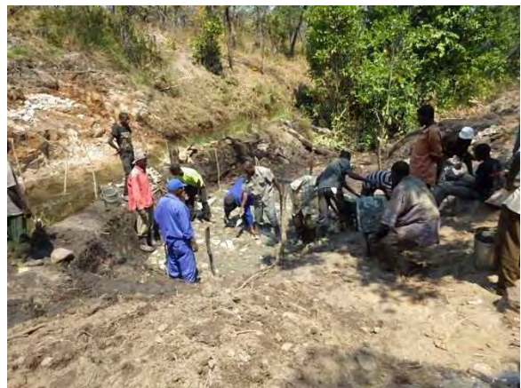
Stone masonry work for apron: Stones are placed and mortar is filled into voids completely. LWG 5-2 Mufili Chibwale. September 12, 2014.
