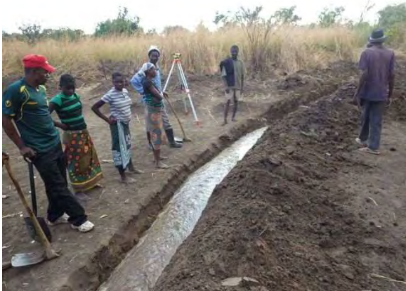
River diversion: Cofferdam was completed and the river water was diverted. NKD 1-3 Musanza. August 18, 2014
