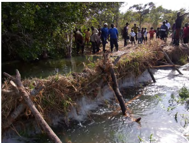
Field Practice on Simple Weir Construction: One of the advantages of this kind is not to completely hold water, enabling water continues to flow.
