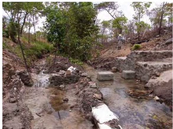
Installation of intake stop-log frame: Right side abutment was almost completed and started construction of intake. Intake stop-log was installed. October 17, 2014.
