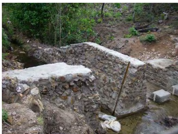
Intake part: Stone masonry for intake canal wall was completed. Stop log frame of intake. Remaining work is left side slope protection and partial improvement of canal. LWG 5-2 Mufili Chibwale. November 20, 2014
