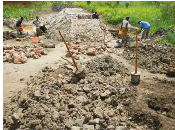
Rammer for compaction of embankment: Embankment is compacted with rammer. MPK 1-17 Lubanga. November 28, 2014.
