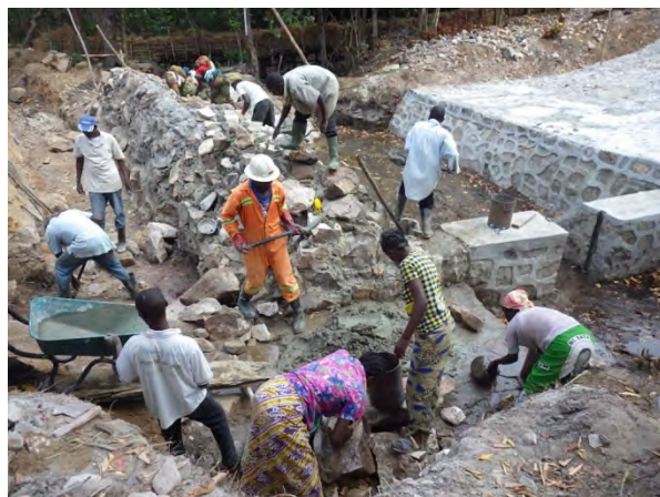
Stone masonry work for intake in Musanda scheme in Kasama district. Masonry group, mortar mixing group and stone ferrying group.
