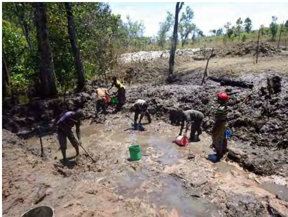
De-watering by buckets: Buckets are used for de-watering if water leakage from the coffer dam is not so large. MPR 14-1 Mpela. September 10, 2014.
