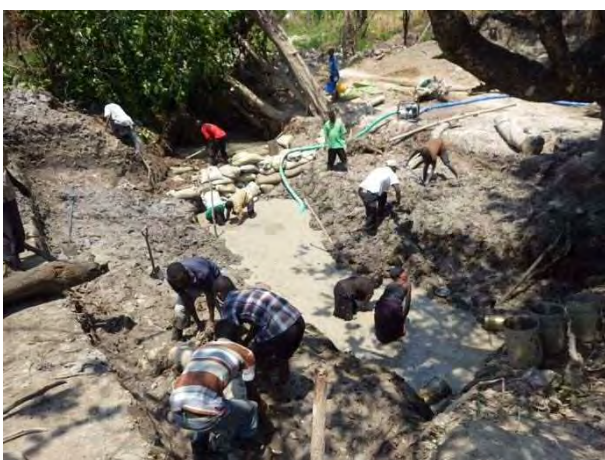
Excavation of foundation: excavation of foundation was difficult due to ground water. Two engine pumps were mobilized for de-watering. Munyele, Nsama. October 10, 2015.
