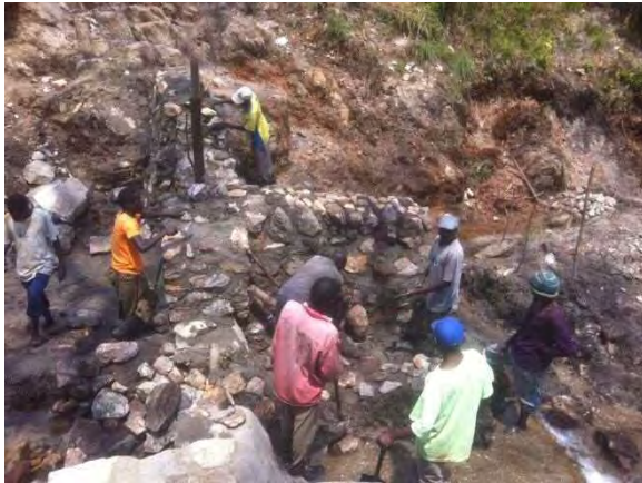
Construction of left side abutment and intake: Stone masonry work for left side abutment and intake. During construction, water flow is diverted to main stream. LWG 5-2 Mufili Chibwale. October 30, 2014.
