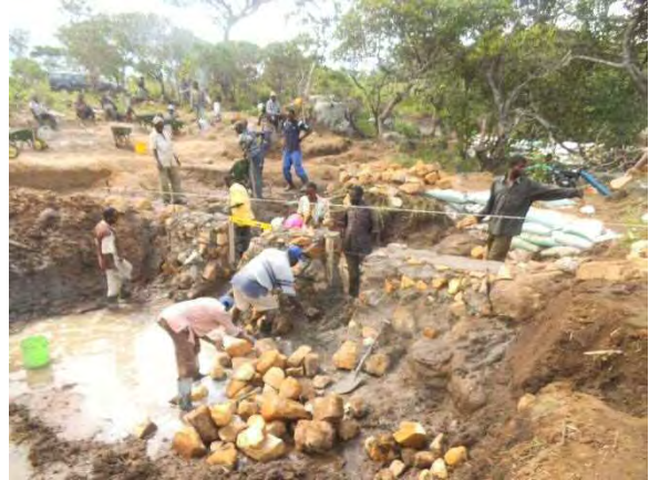
Construction of spillway section of stone masonry weir: Main part of spillway is constructed with stone masonry. MBL 2-7 Kawama. November 27, 2014.
