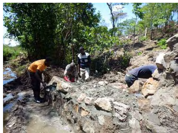
Stone masonry work for intake canal: Upstream end of intake canal is built strongly to avoid erosion by river flood water. LWG 5-2 Mufili Chibwale. November 14, 2014.
