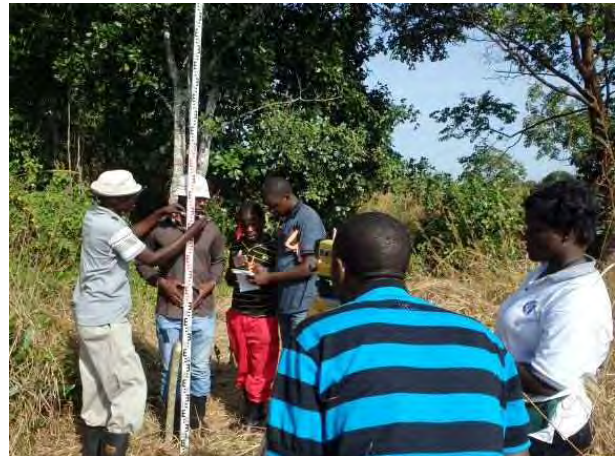
Preparation Work: Even in the method to stand the staff gauge, the participants of TSB training confirmed to survey the topographic condition correctly.
