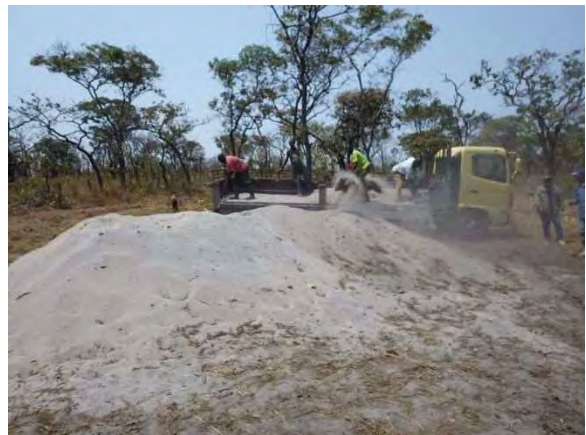
Sand Ferrying: Sand was ferried from the borrow pit about 5km away from the site. LWG 5-2 Mufili Chibwale. September 5, 2014
