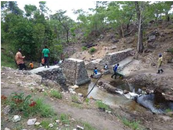
Upstream view of the weir: Main part of stone masonry weir was completed. LWG 5-2 Mufili Chibwale. November 11, 2014.
