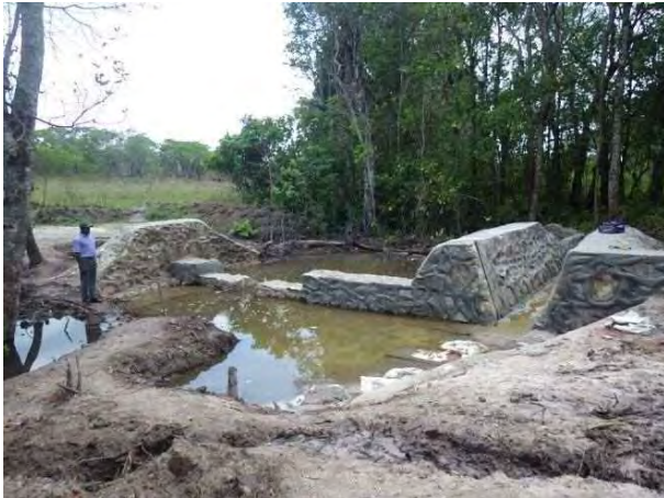
Upstream view of the weir: Main part of stone masonry weir was completed. Remaining work is left side embankment and a part of canal lining. MPR 14-1 Mpela December 1, 2014.
