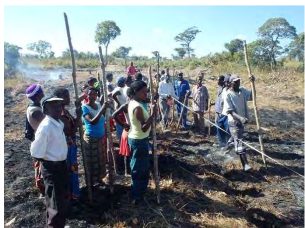
Site clearing and putting pegs: Trees, grass, roots and surface soil were removed and pegs were put. Kalila, Mansa. July 8, 2015
