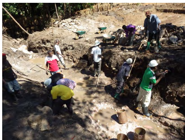
Excavation for foundation of apron in Musanda scheme in Kasama district. Using buckets for de-watering. There are big stones in the river bed.
