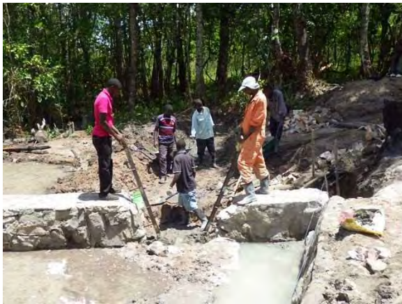
Installation of intake stop-log frame: Steel intake stop-log frame was installed. MPR 14-1Mpela. November 13, 2014.
