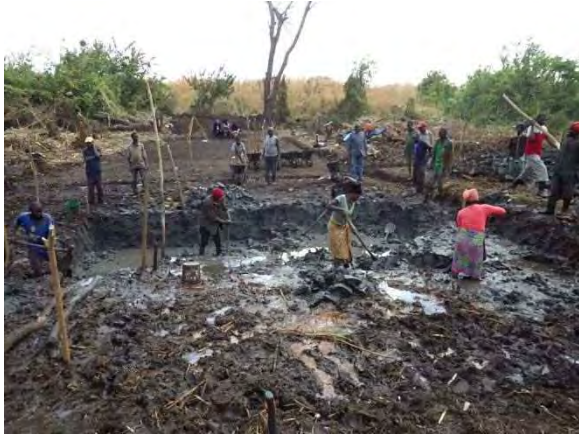
Excavation for foundation of apron: Excavated to solid foundation. Excavation for foundation of apron was done with hoes, shovels, pick axes, and de-watering by buckets. MPK 1-17 Lubanga. August 15, 2014
