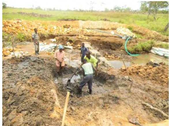
Excavation of intake part : Intake part is excavated to required elevation. MBL 2-7 Kawama. November 28, 2014.
