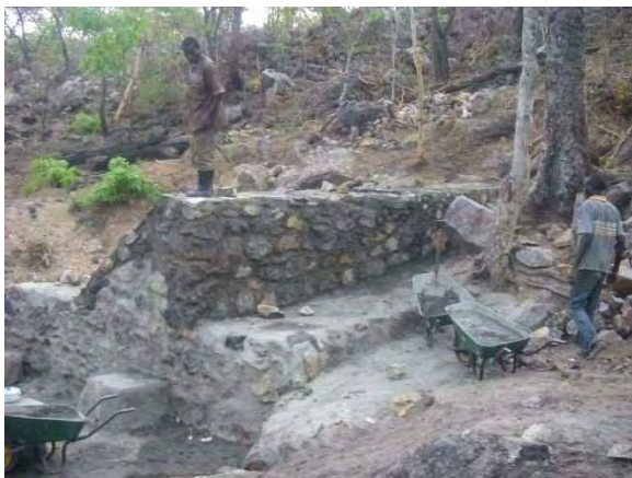
Completed right side abutment : Right side abutment was completed up to required elevation. LWG 5-2 Mufili Chibwale. October 27, 2014.
