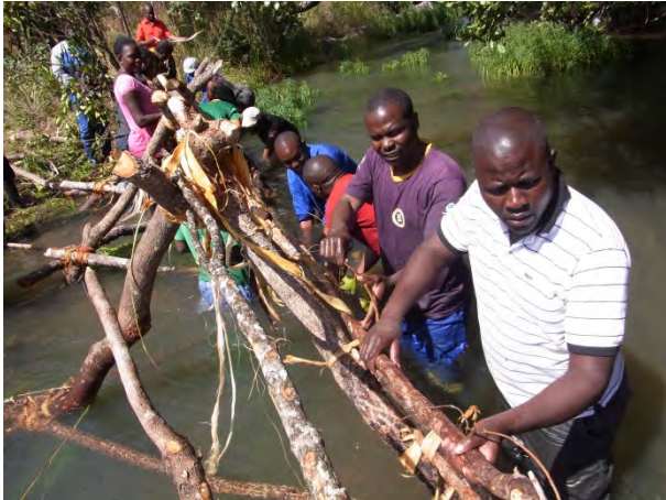
Field Practice on Simple Weir Construction: horizontal members are placed across the trigonal props so as to connect them and stabilize the structure.
