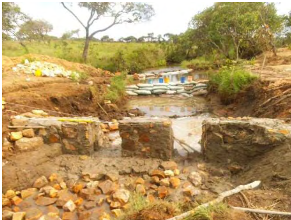
Completed spillway with stop log : Spillway with stop log frame was completed. MBL 2-7 Kawama. November 28, 2014.
