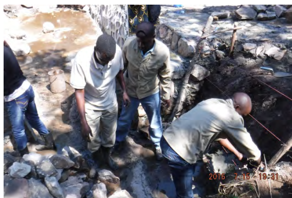
TSB participants practically learned how to construct weir body at actual construction site in Kasama
