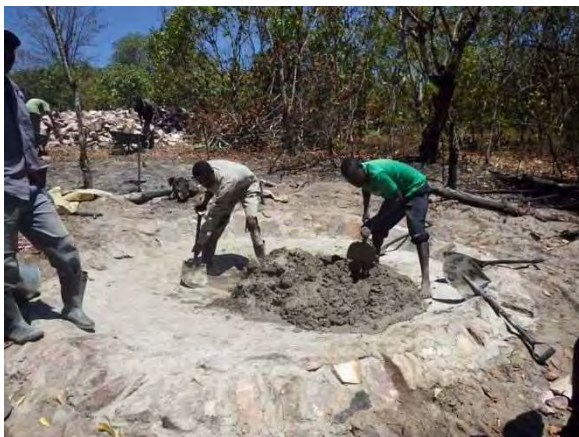
Mortar mixing: Mortar is mixed in the prepared mortar mixing place. MPR 14-1 Mpela. September 16 2014.
