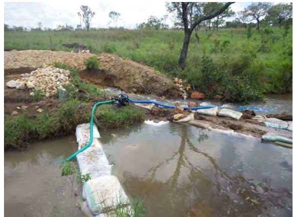
De-watering by engine pump: Engine pump was introduced for de-watering due to a lot of water leakage from the coffer dam. MBL 2-7 Kawama. November 26, 2014.
