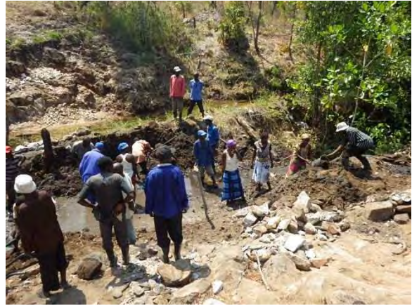
Excavation for foundation: Mud and soft soil on the rock foundation was removed. LWG 5-2 Mufili Chibwale. September 12, 2014.
