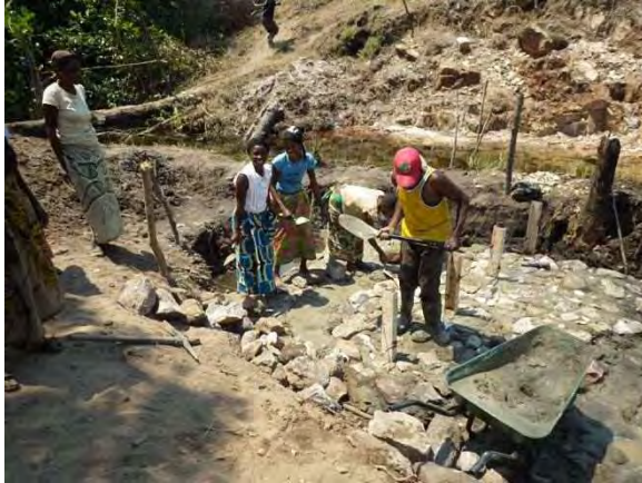
Installation of spillway stop-log frame and stone masonry work for apron.: Steel stop-log frame was installed. Ladies also worked for stone masonry work. LWG 5-2 Mufili Chibwale. September 17, 2014.
