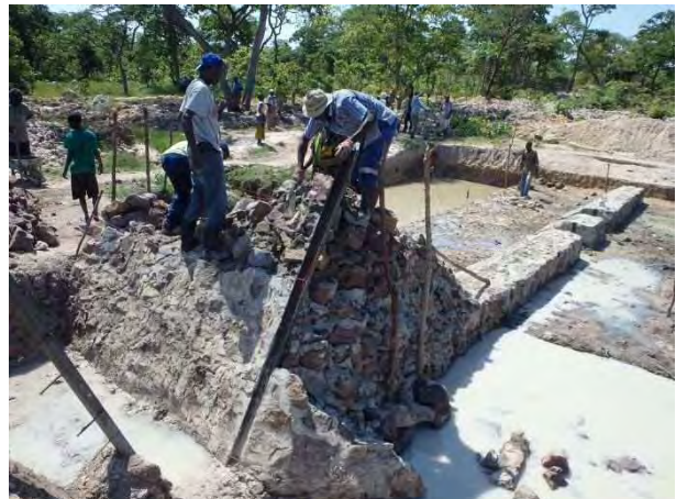
Construction of Right side abutment: Stone masonry works for left side abutment is constructed. Kalila, Mansa. November 19, 2015
