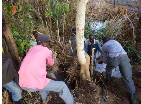
Construction of coffer dam: Constructing coffer dam with simple weir technique.. NKD 1-3 Musanza. August 18, 2014
