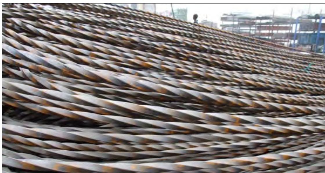
Figure 9: Kenyan Rebar - Mostly Twisted rather than Deformed
