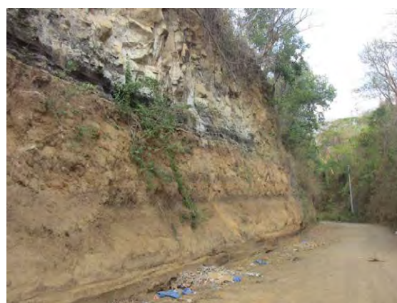
Some side slopes along an upper stretch of cauce are unsteable and frequently collapse. The slope set back two meters to land side.
