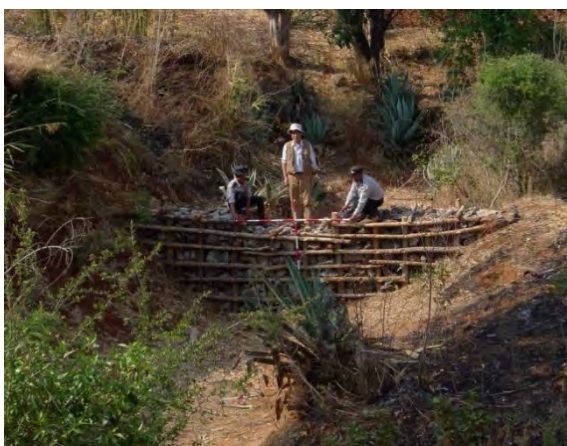
Photo II -14 Catchment dam build by Forest Department (Utilization of rocks and timbers locally procured)
