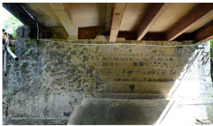
Steel H girder and expanded by T girder, Substructure is Stone Masonry
