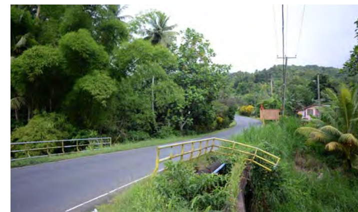
Steel handrail are damaged/inclined
