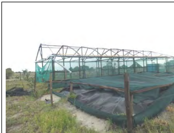
February 02 nd 2017, at Okatana, under replacement of roof sheets for roof water harvesting.
