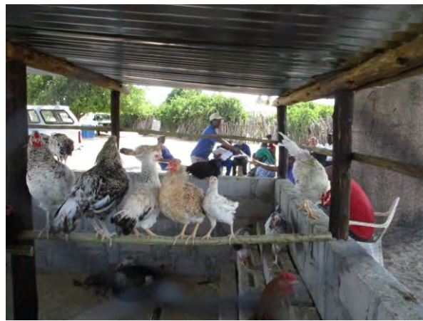
Improved chicken house constructed by the support of N-CLIMP at Tsandi (Chicken) in Omusati (Shot at 3rd Training for Farmers Group on Feb. 8 2016)
