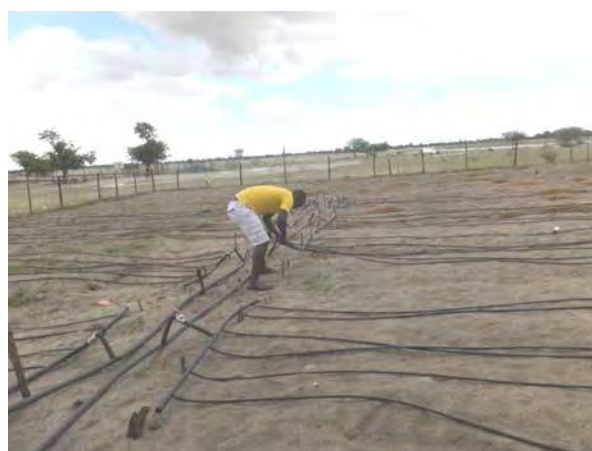
Feb. 02 nd 2017, installation of drip irrigation system at Okatana Constituency in Oshana Region, by replacing with the deteriorated one.
