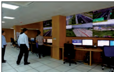
Figure 6-22 Traffic Control Center
