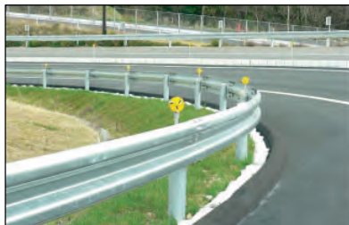
Figure 6-21 Delineator Attached on Guard Rail
