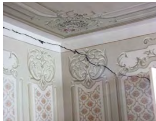
Situation of damaged house
