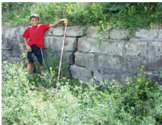
Deformation of retaining wall
