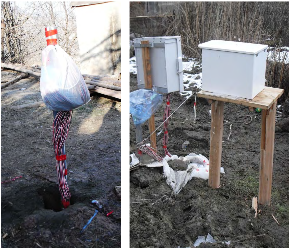
Figure 3.2.4: Installation of a PVC pipe affixed to the sensors into the borehole to record ground water levels and deformation data
