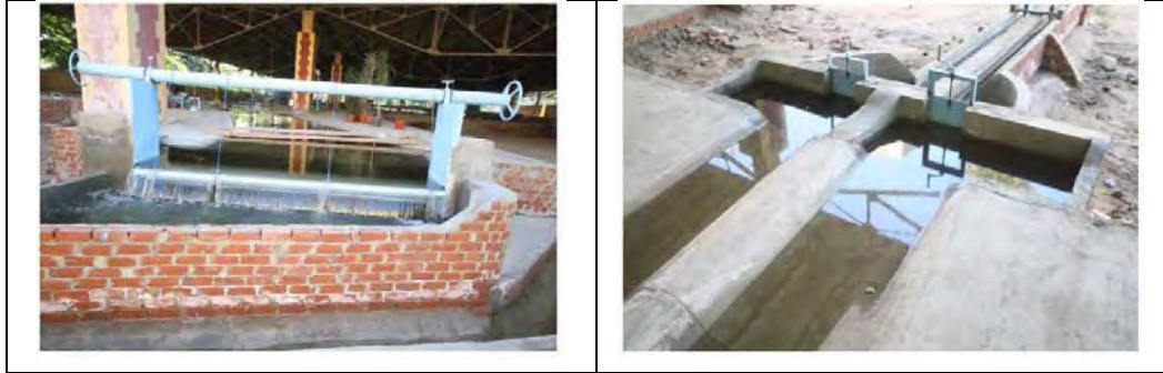
Figure 3-2.3 Discharge measuring device (regulator)
