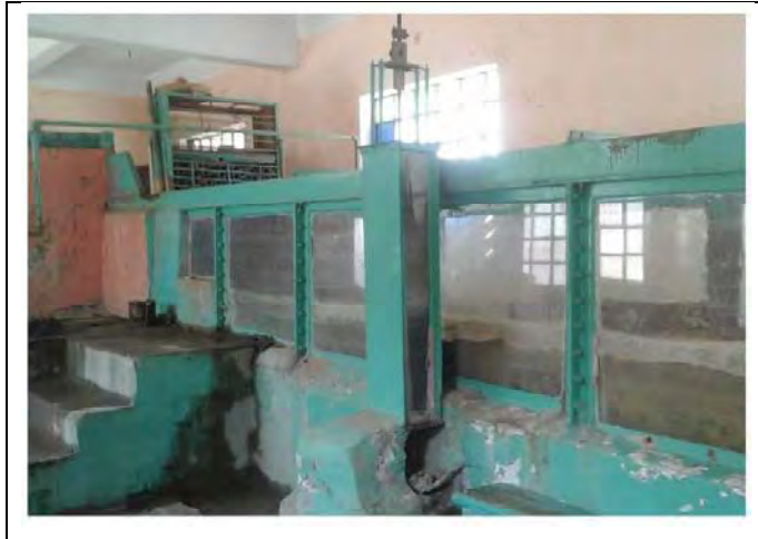
Figure 3-3.4 Water level measuring equipment (point gauge)
