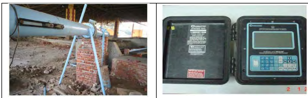
Figure 3-2.2 Inflow measuring equipment (ultrasonic flow meter)
