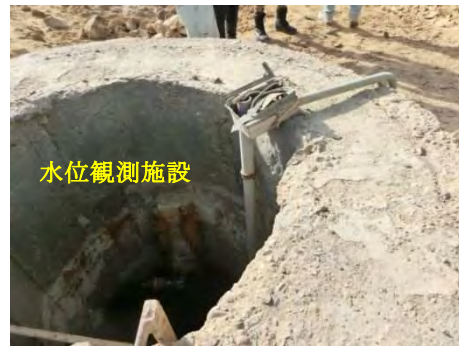
Water Level Monitoring Facility
