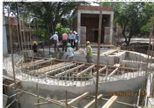
SARAIYA PUMPING STATION - P2
