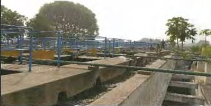
Note) 4-Dec-2015 MirzapurSTP-3 UASB Reactor
