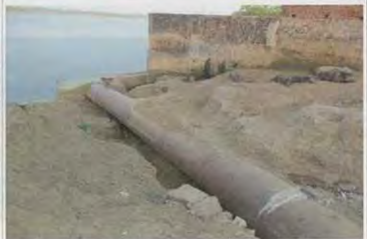
Note) 30-Sep-2015 Varanasi NagwaPS-6 Transmission Pipe to Ramna proposed STP
