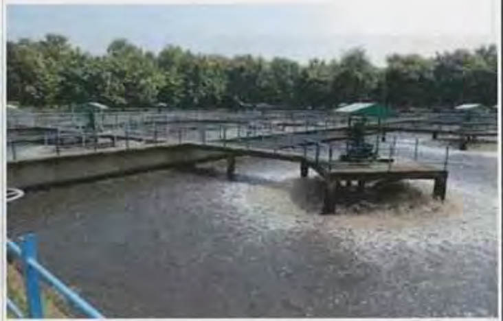
Note) 30-Sep-2015 Varanasi DinapurSTP-2 Aeration Tank
