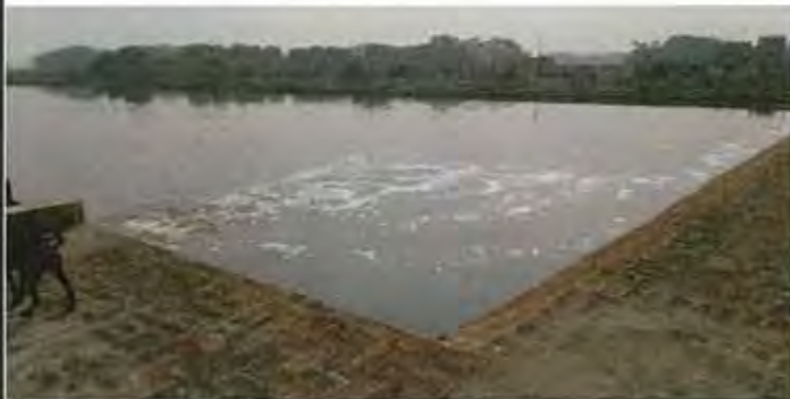
Note) 4-Dec-2015 MirzapurSTP-5 Oxidation Pond
