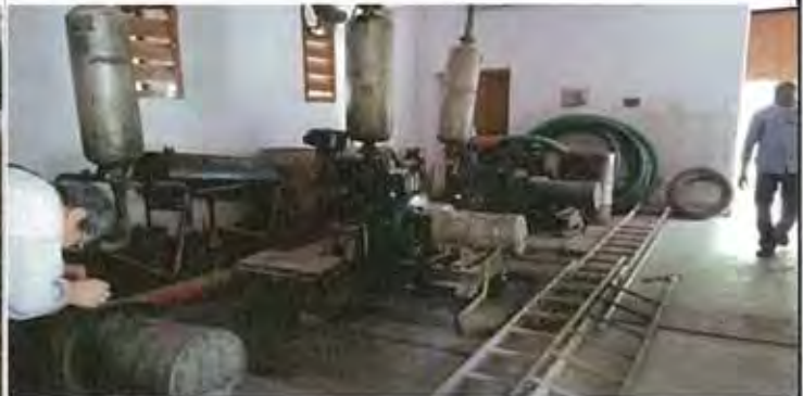
Note) 4-Dec-2015 MirzapurSTP-6 Generation Room
