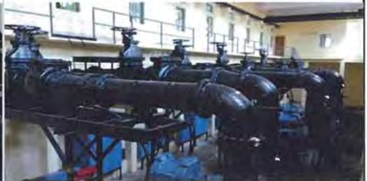
Note) 30-Sep-2015 Varanasi KoniaMPS-6 Transmission Pipe
