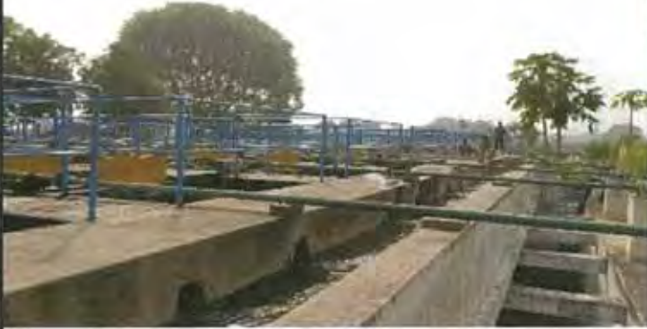
Note) 4-Dec-2015 MirzapurSTP-3 UASB Reactor
