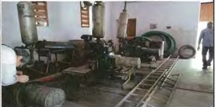
Note) 4-Dec-2015 MirzapurSTP-6 Generation Room
