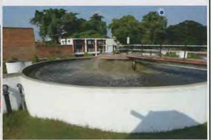
Note) 30-Sep-2015 Varanasi BhagwanpurSTP-4 Aeration Tank
