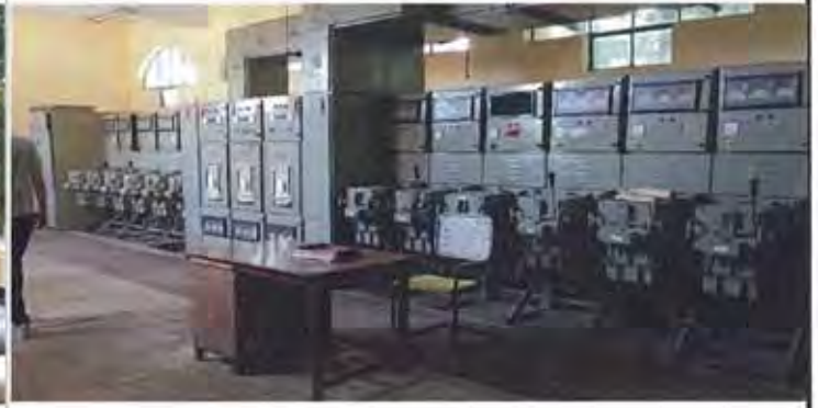
Note) 30-Sep-2015 Varanasi KoniaMPS-2 Electrical Room
