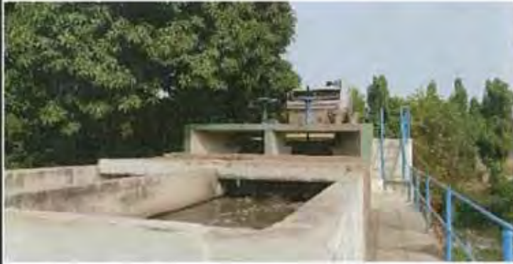
Note) 4-Dec-2015 MirzapurSTP-1 Grit Chamber
