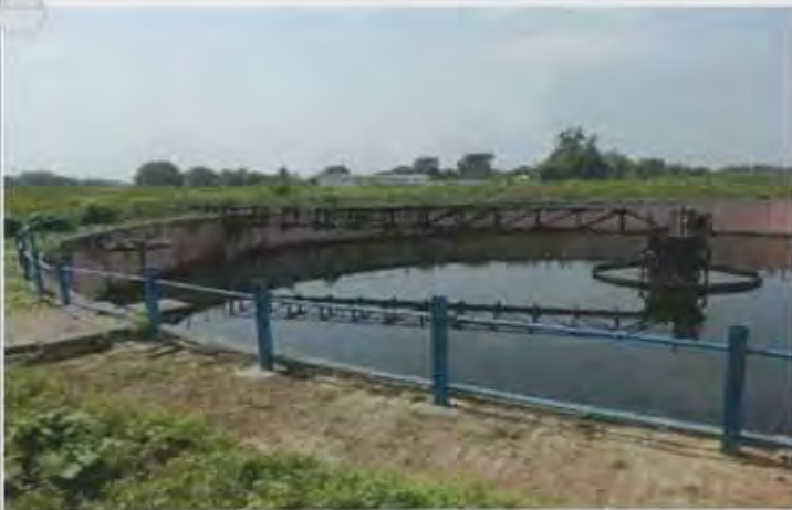
Note) 30-Sep-2015 Varanasi DinapurSTP-3 Primary Sedimentation Tank
