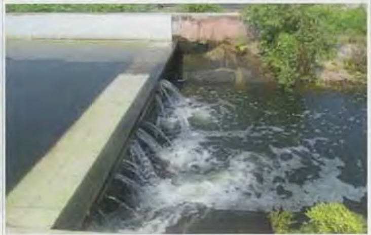
Note) 30-Sep-2015 Varanasi DinapurSTP-6 Outlet Channel
