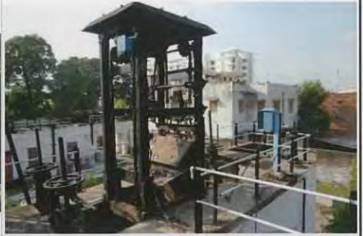
Note) 30-Sep-2015 Varanasi BhagwanpurSTP-2 Screening unit
