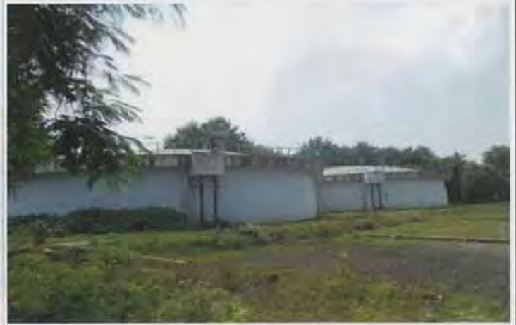
Note) 30-Sep-2015 Varanasi DinapurSTP-4 Digester Tank
