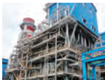
Heat Recovery Steam Generator
