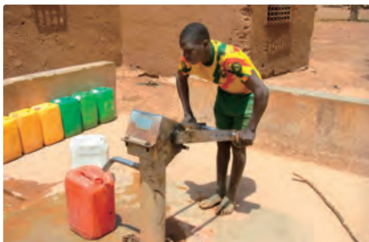
Deep well with hand-pump facility
