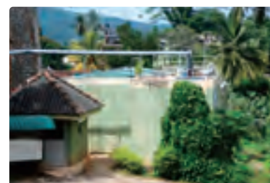
③ Waste water treatment facility installed at a hotel utilizing the sub-loan from this project
