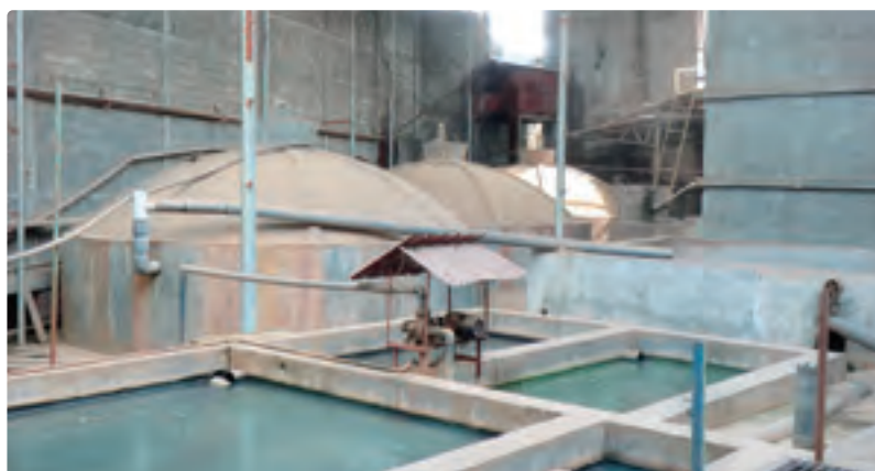
① Waste water treatment facility installed at a rice mill utilizing the sub-loan from this project
