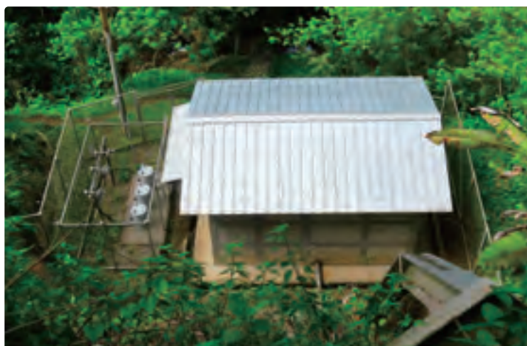
Power generation facility (Seasir). The penstock entering the facility can be seen in the front
