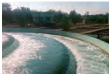
Water Treatment Facility (T.K. Halli)
