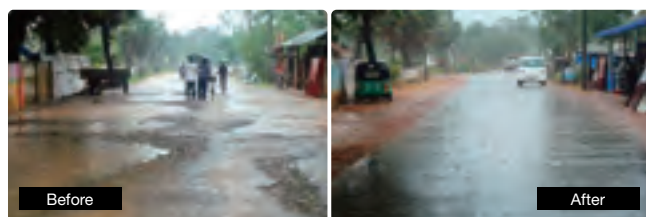
Before and after the road rehabilitation (photo provided by the implementing agency)
