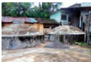
② Waste water treatment facility installed at a rice mill utilizing the sub-loan from this project
