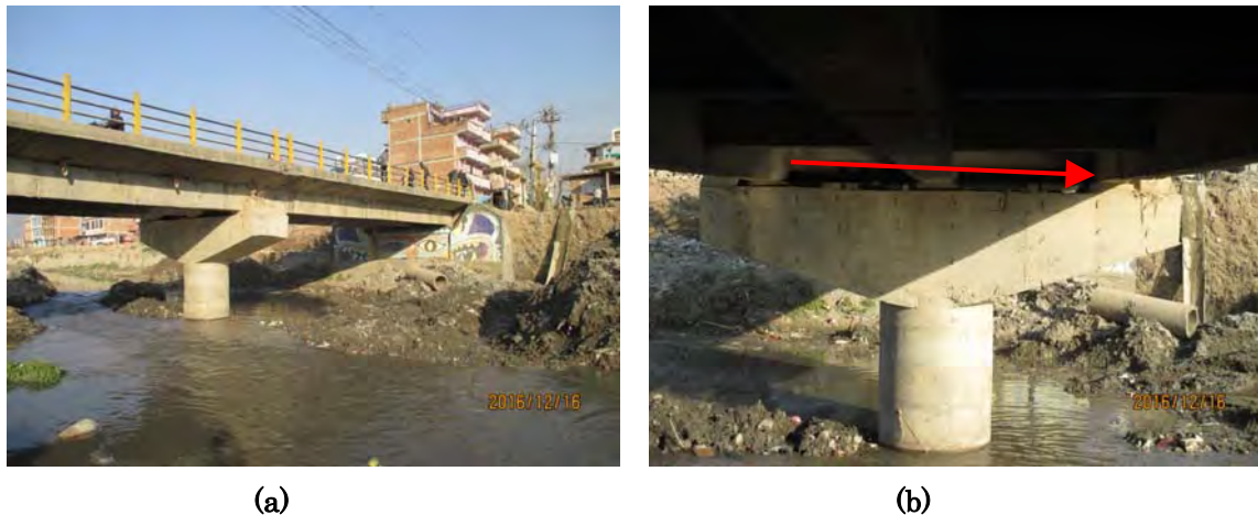
Figure 5.4.5 Damage Situation in No.94 Bridge
