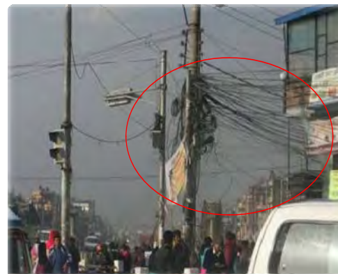
Unsafe overhead cabling on sidewalk
