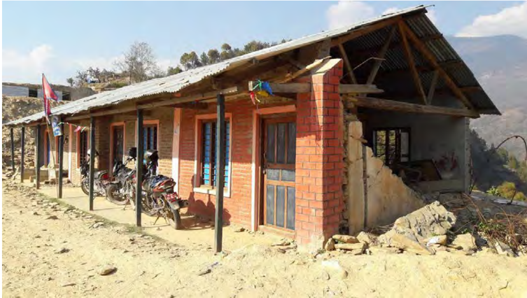
Photo 1: Damaged building at Kamaladevi L.S School
