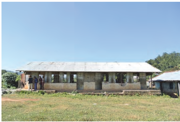
School site visit in Nuwakot District (Building damage assessment) October 27, 2016
