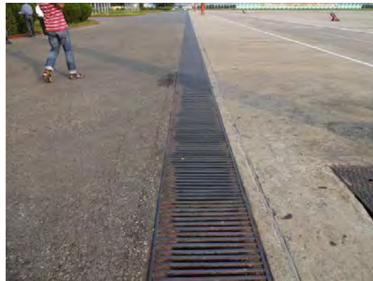
Existing Ditch with Grating
