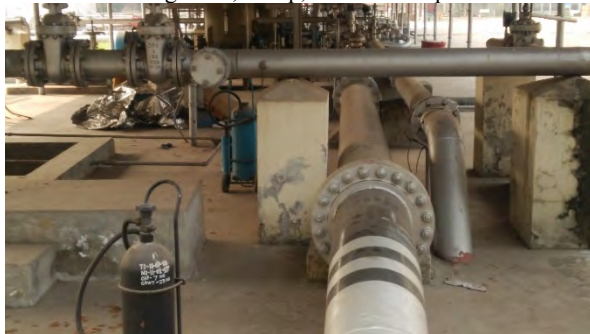
14-inch and 8-inch Hydrant Pipes
