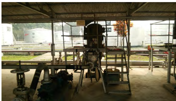
Existing Tank, Pump, and Filter Separator
