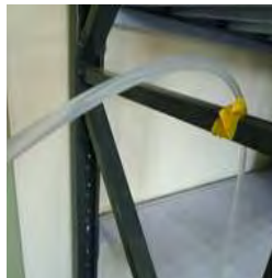
Incorrectly Fixed; the pipe gets squashed by its own weight where it is fixed.
