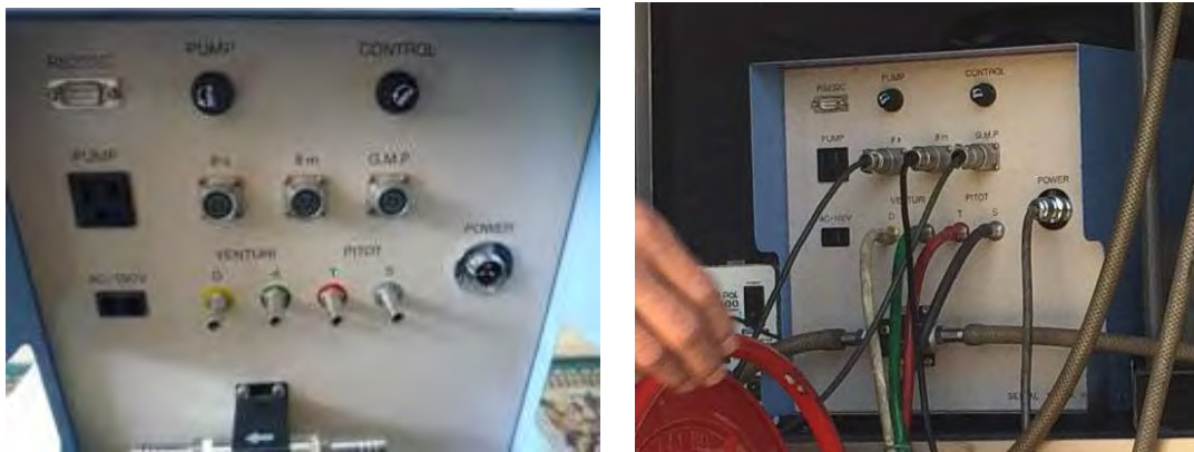
Figure 8-10 Installation of Automated Dust Sampling Instruments
