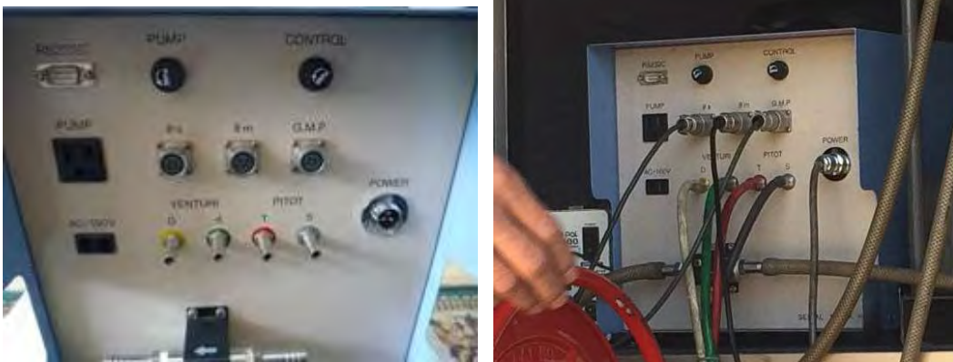
Figure 5-5 Installation of Automated Dust Sampling Instruments
