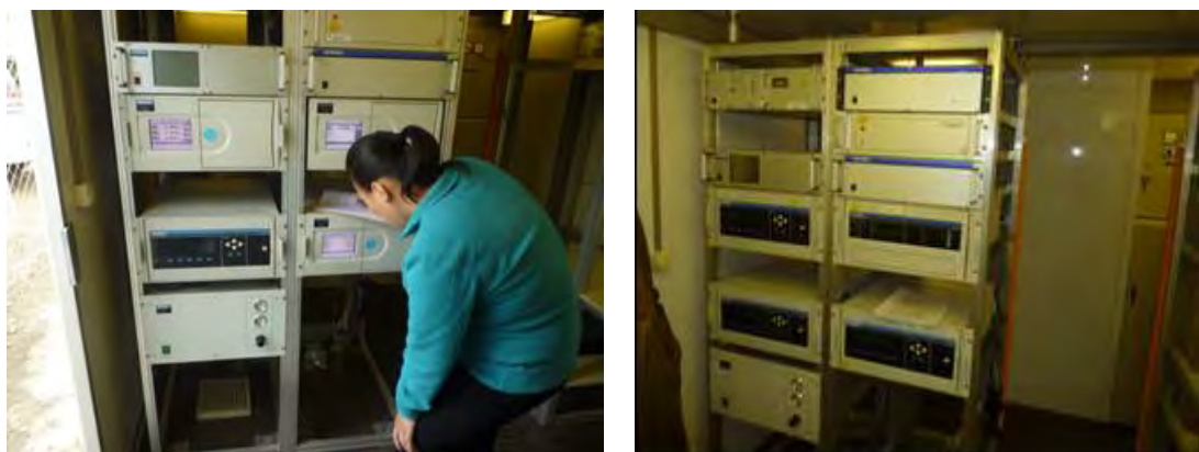
Figure 2.1-1 Stationary Air Quality Monitoring Station
