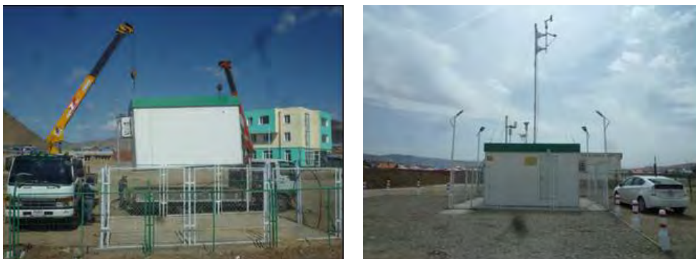
Figure 2.1-3 Established New AQMS
