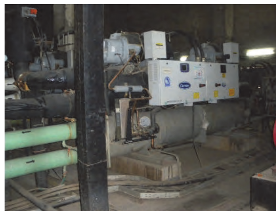
Figure 6.2.38 Centrifugal chiller (Mahatma mandir, Gandhinagar)
