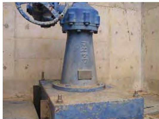
Picture 5-2-9 Sand Flush Gate Winch
