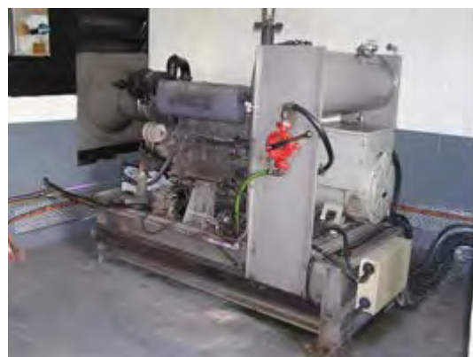
Picture 5-4-2 Diesel Generator
