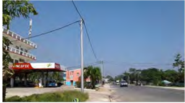
Picture 5-6-4 Luganville City Domestic Low Voltage Distribution Line
