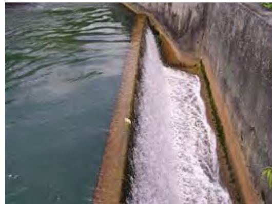
Picture 5-2-13 Headtank Spillway Overspill Condition
