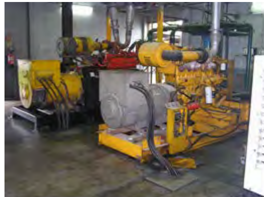
Picture 5-3-2 Diesel Generator
