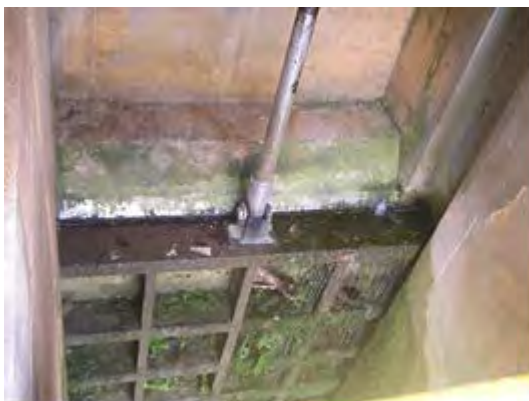
Picture 5-2-8 Sand Flush Gate
