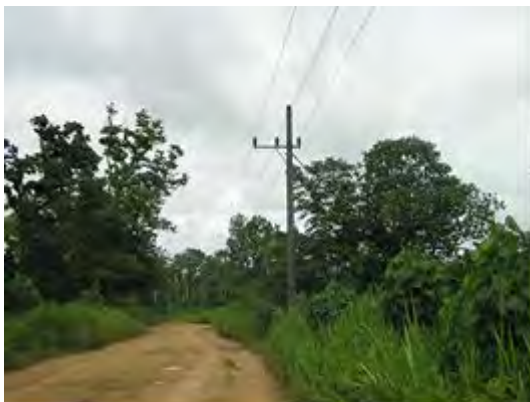
Picture 5-6-1 20kV Transmission Line (Sarakata Hydro. ~Luganville)
