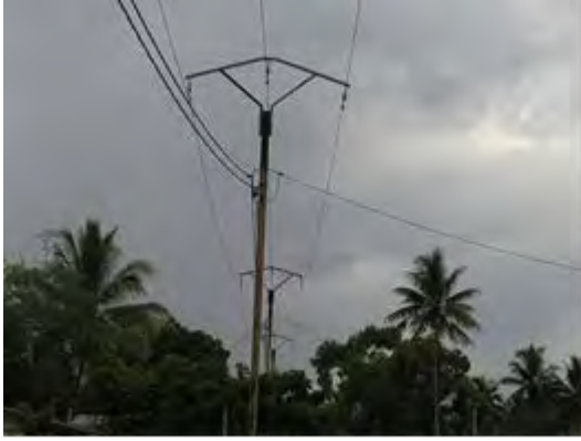
Picture 5-6-3 5.5kV Distribution Line (Low Voltage Distribution Line Coexistence Section)
