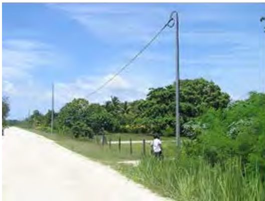
Picture 5-6-5 Newy Extended Low Voltage Distribution Line (Near Million dollar point)
