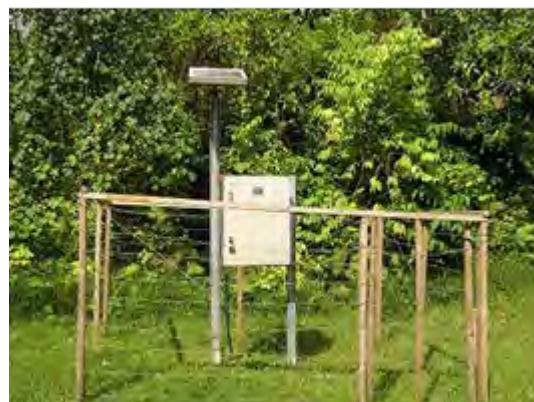
Picture 5-2-4 Automatic Water Level Gauge Recorder
