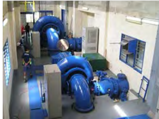
Picture 5-2-17 Hydroelectric Power Equipments
