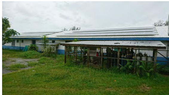
Picture 5-5-1 Solar Equipment of Hospital (20kW)
