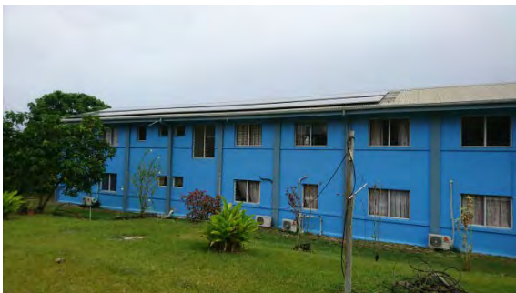
Picture 5-5-2 Sanma Province Office(10kW)
