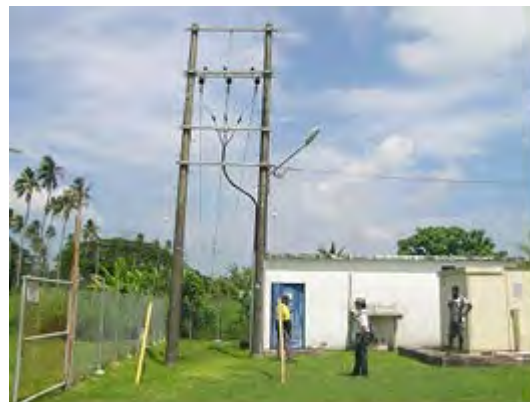
Picture 5-6-2 20KV/5.5kV Luganville Substation
