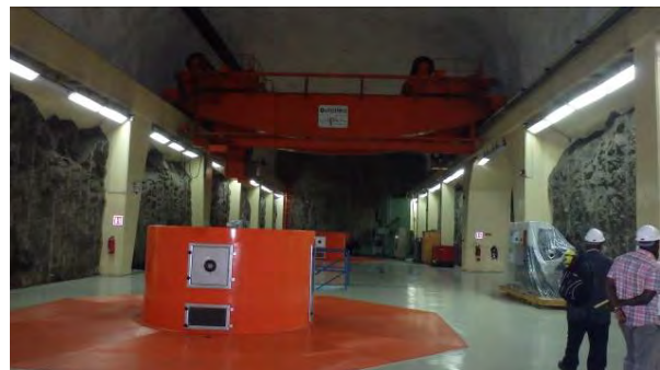
<Generator Floor in Underground Powerhouse>
