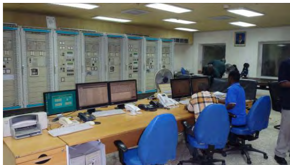
<Control Room in Underground Powerhouse>
