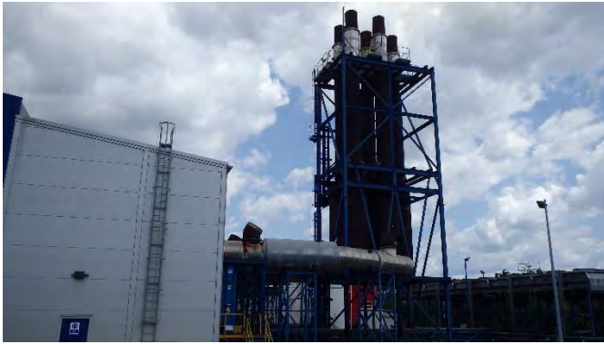
< Overview of the plant >
