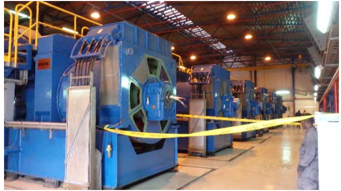
< Gas Engine Unit (Wärtsilä W20V34SG)>
