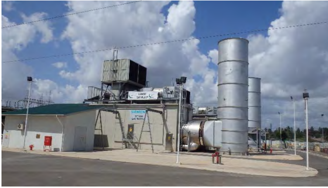
<Overview of the plant>
