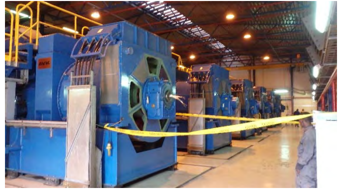
<Gas Engine Unit (Wärtsilä W20V34SG)>
