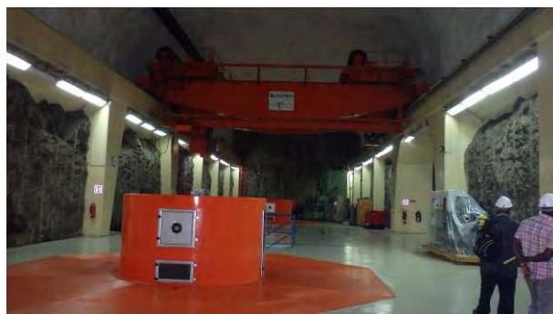
<Generator Floor in Underground Powerhouse>
