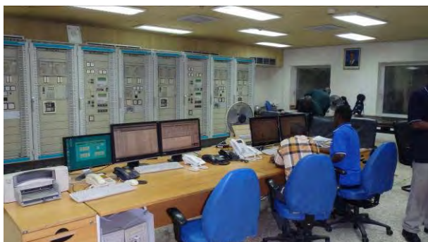
<Control Room in Underground Powerhouse>
