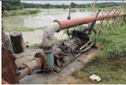
Figure 4.4.5.1 Sand booster pump
