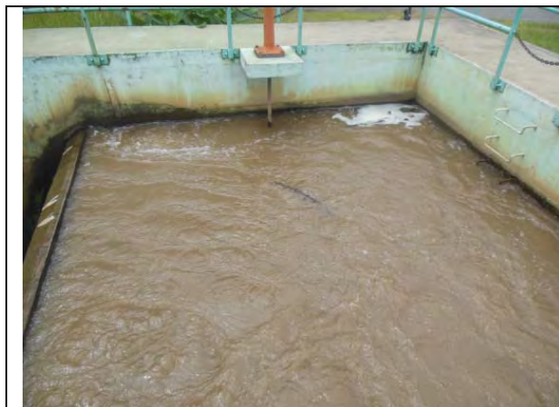
Inflow at plant entrance (high turbidity)
