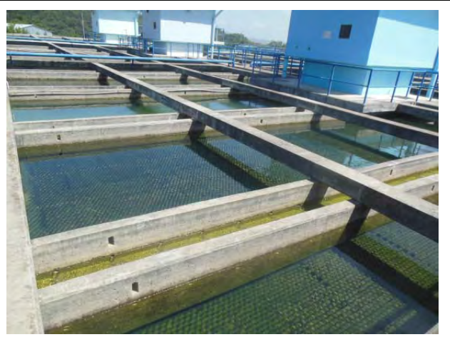
Sedimentation tanks with settling plates
