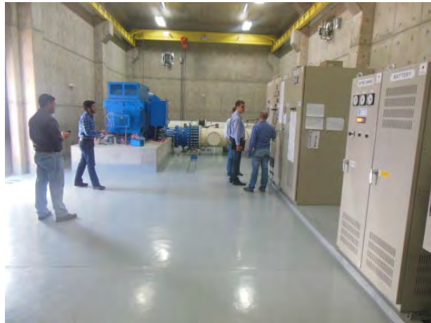
Micro hydropower generation station
