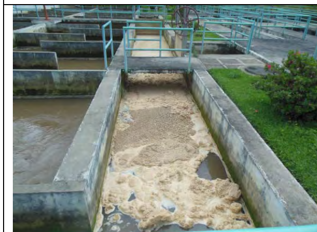
Sedimentation tank (much scum due to high concentrations of detergent in the raw water)
