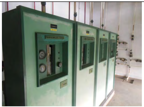
Chlorine dosing controller (two out of the four were not operational at the time of the visit)
