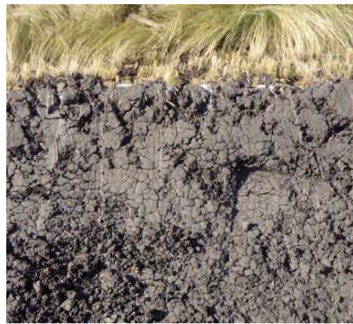
Photo: Expansive soil in the dry condition (CBR investigations may sometimes show high readings.)
