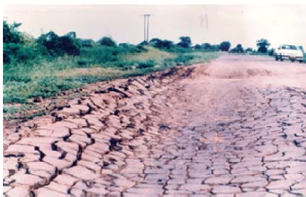
Cracking and rutting due to the lack of pavement thickness
