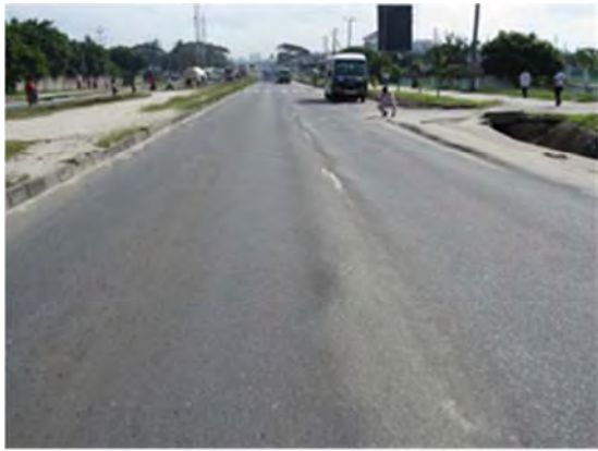
Tanzanian case: Rutting occurred at the flat section of the urban trunk road. Surface layer “flows” to the center.
