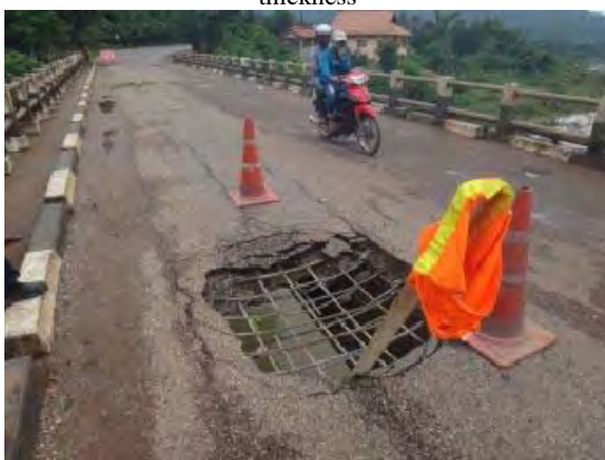
A pothole in a concrete slab
