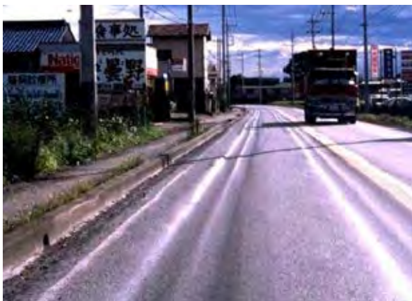
Rutting caused by overloaded vehicles
