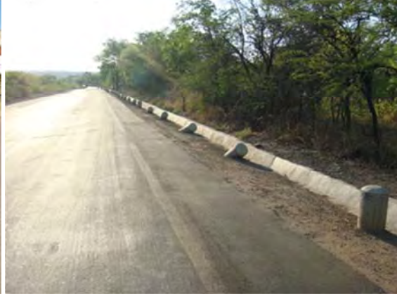
Zambia: Livingstone Road before repair (Extreme breathing)
