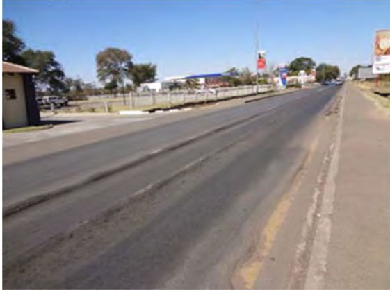
Zambia: Livingstone Road before repair (Extreme rutting)
