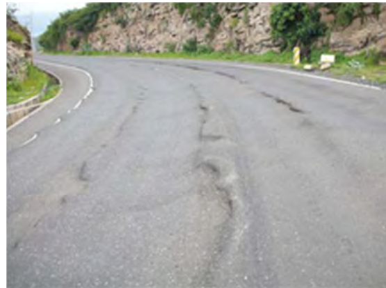
Ethiopian case: Rutting occurred at a steep curve section of a rural road in precipitous mountains. Surface layer flows to the inside of the curve.
