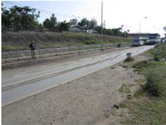
Photo: Ethiopia; Main city road Bearing capacity of the lower road section deteriorated by expansive soil (black cotton soil) leading to rutting of the surface.
