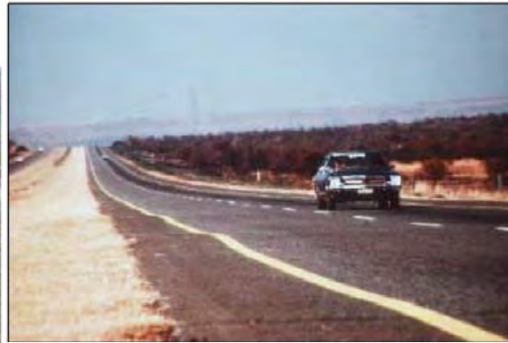
Photo: South Africa; Road surface over a culvert raised by expansive soil Source : SAPEM Chapter-6
