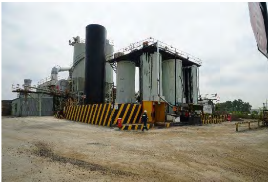
SA: Continuous plant for Much Asphalt (the largest asphalt supplier in SA)
