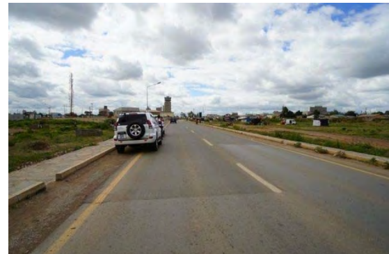
Zambia: Condition of “Tokyo way” in Lusaka (Fair: Repaired section after 7 months (a rainy season))
