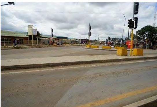
Zambia: Condition of “Tokyo way” in Lusaka (Fair: Repaired section after 7 months (a rainy season))
