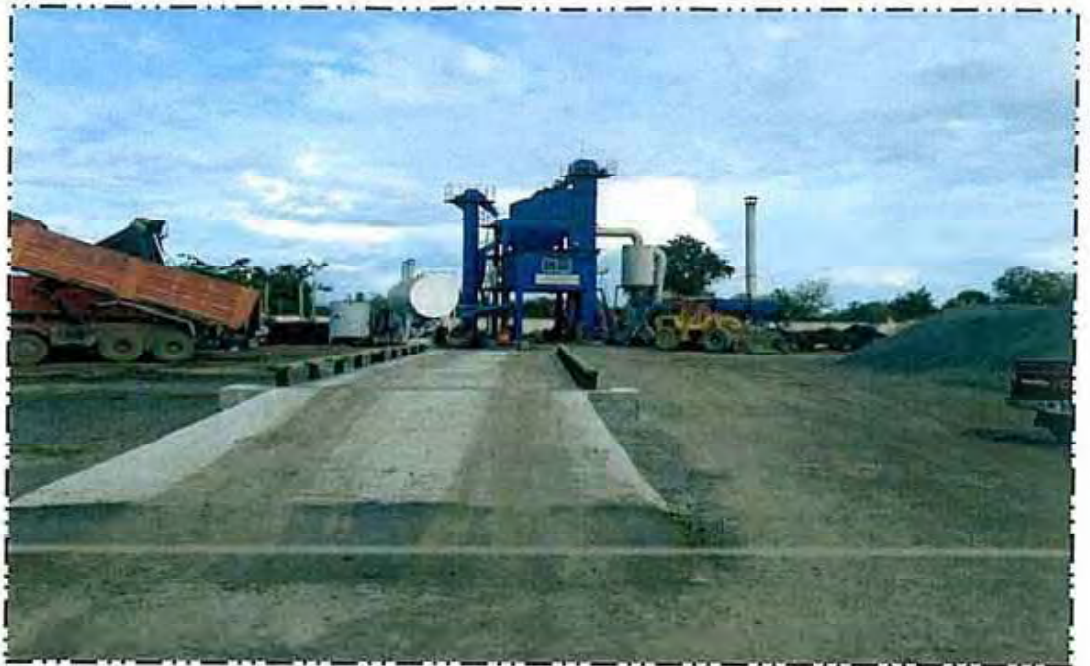
Asphalt plant Machinery
