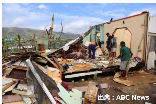
Figure 3 Damage situation by Winston (Fiji)
