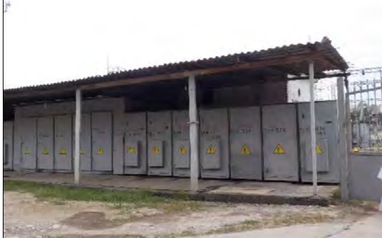
10kV distribution switchgears
