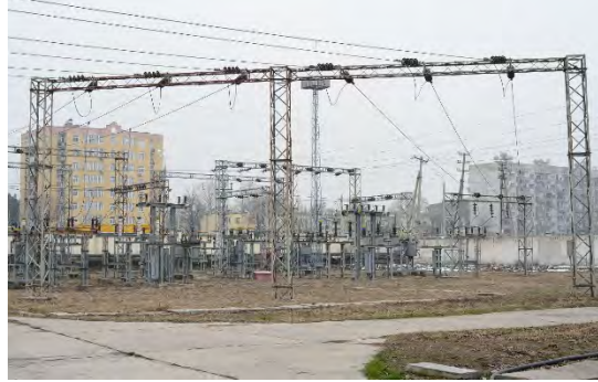
35kV switchgears and support structure
