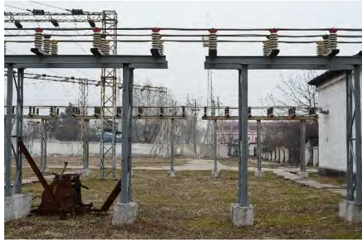
10kV busbar conductor
