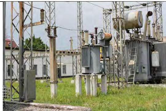
25MVA transformer and busbar conductor to 10kV distribution switchgear building
