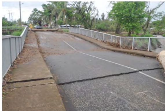
Figure 10 Damaged Bridge on Faatoia Road
