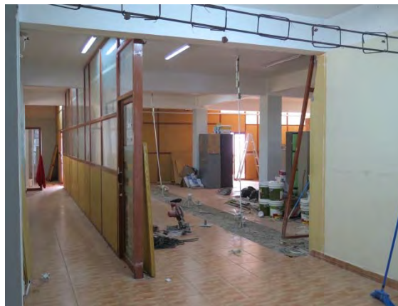
Under reformation of GDMR office Server room designed at Right, overside
