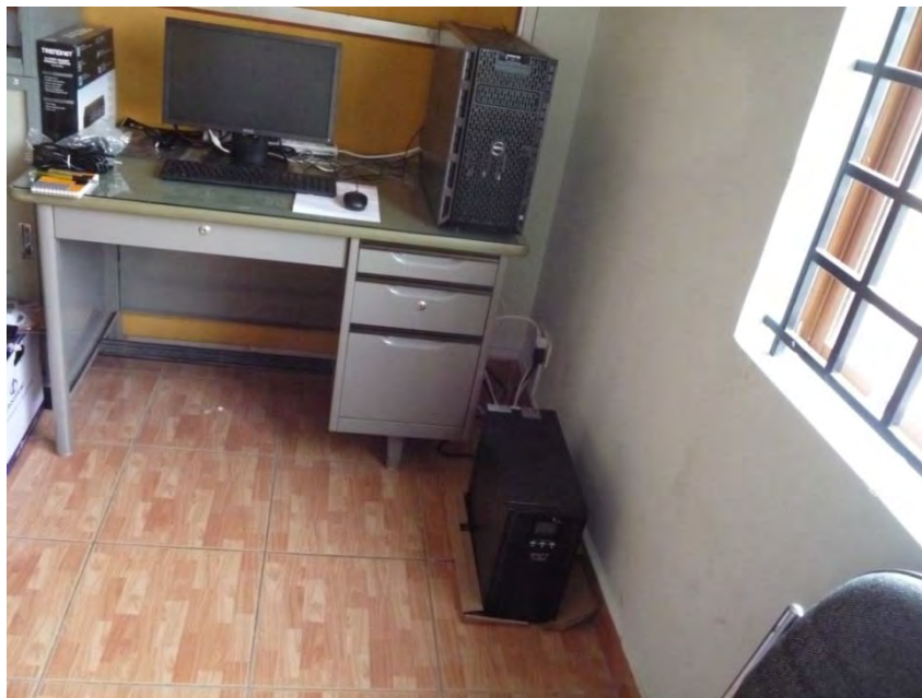
Server PC (on desk) and UPS (at floor), in Server room of GDMR office
