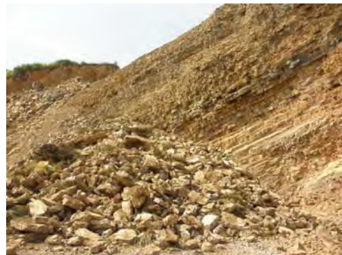
Condition of the remained high-wall There are a lot of joints and cracks
