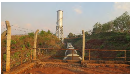
5) Penstock and Surge Tank
