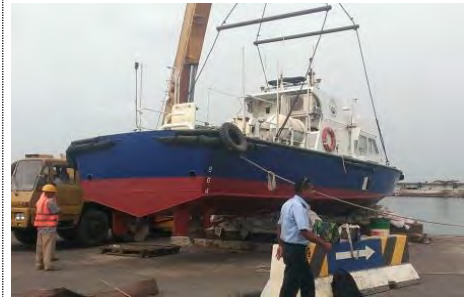
Hoisting Patrol boat for launching after the completion of Installation Work of DHSDAS and Hull/Engine (31 Jan. 2014)
