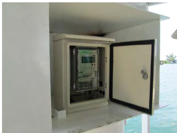
Inside Tide Station. RMD5225WLB-2 Tide Gauge.
